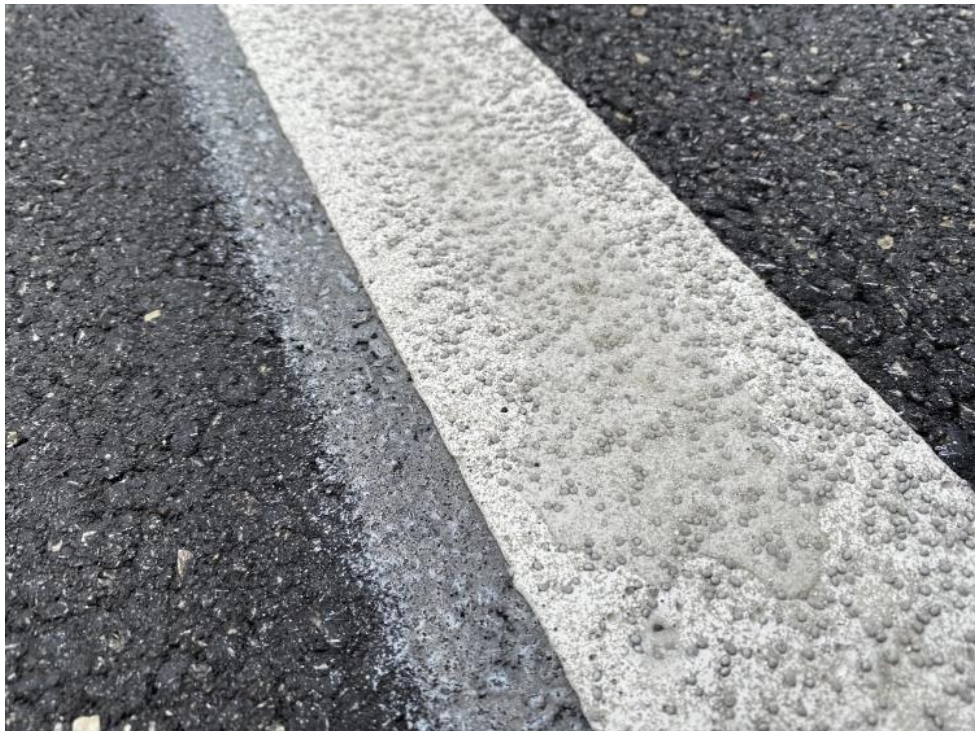
Figure 5. Water Pooling on Marking.
