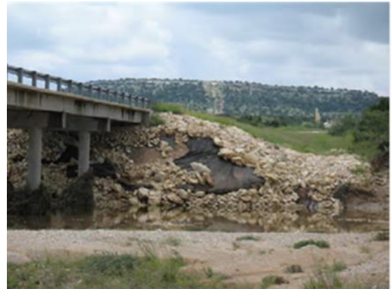
Figure. 1. Riprap Protection and Failure (Courtesy of John Delphia).
