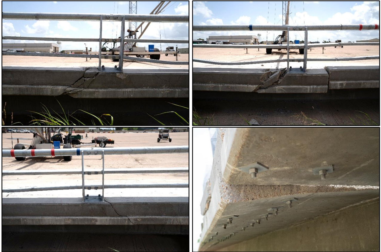
Figure 5.4. Field Side of TxDOT T2P Retrofit Bridge Rail after Test No. 440861-2.
