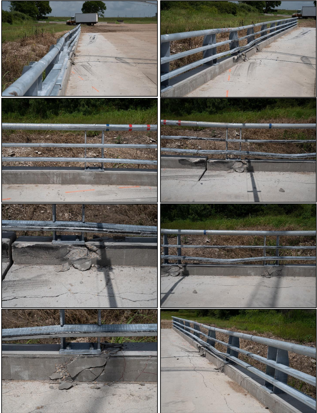
Figure 5.3. TxDOT T2P Retrofit Bridge Rail after Test No. 440861-2.
