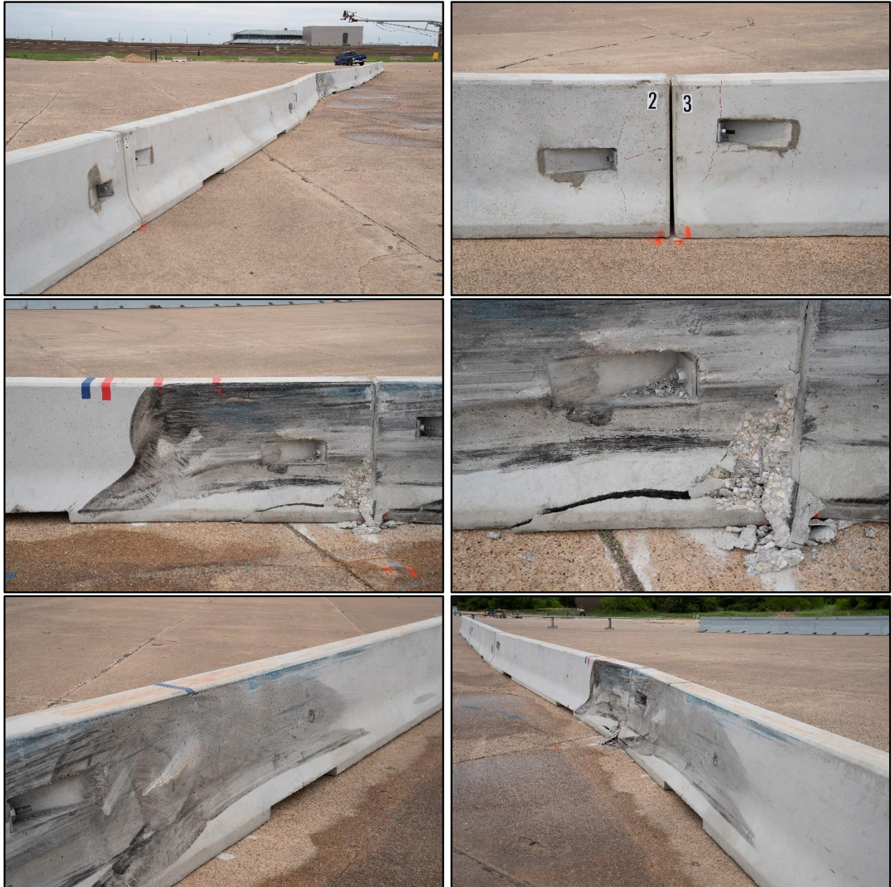
Figure 5.3. F-Shape PCB with X-Bolt Connection after Test No. 440861-01-1.
