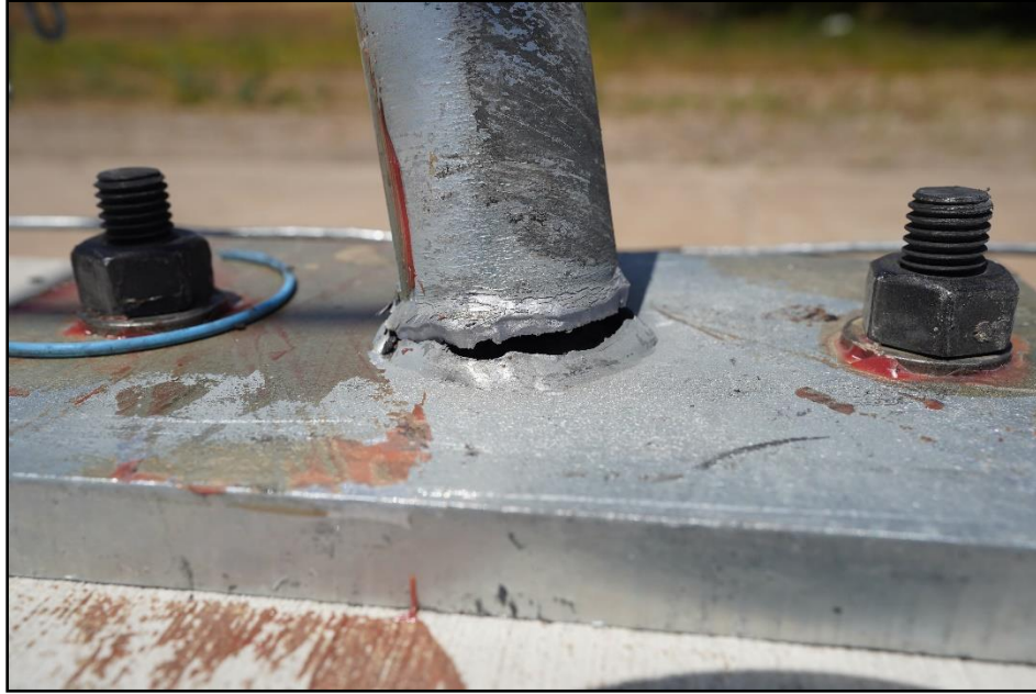
Figure 9.7. Chain-Link Fence on F-Shape Barrier after Test at the Base of Post 6, Test 440822-01-5.
