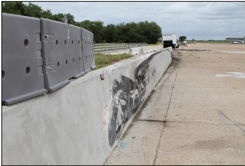
Figure 5.6. Armorcast® Gawk Screen on Single-Slope Barrier after Test at Impact Location, Test 440822-01-1.
