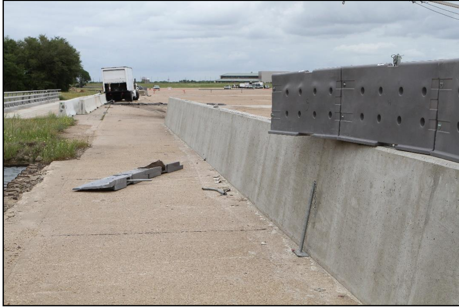
Figure 5.7. Rear View of the Armorcast® Gawk Screen on Single-Slope Barrier Post Impact, Test 440822-01-1.
