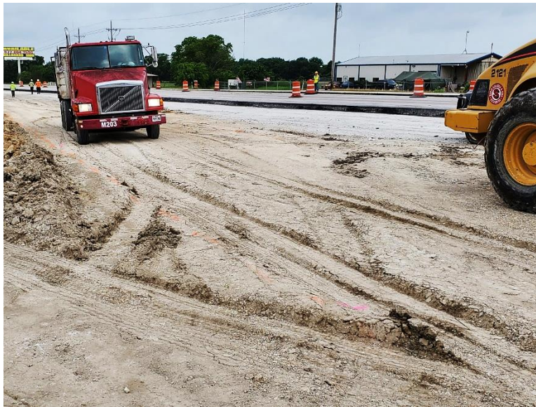
Figure 20. DAL-SH 121 Detour, Soft Subgrade Rutting under Construction Traffic.
