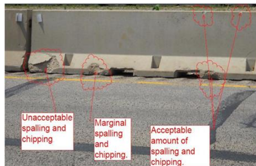
Figure 3.4. Spalling and Chipping—WisDOT (43).
