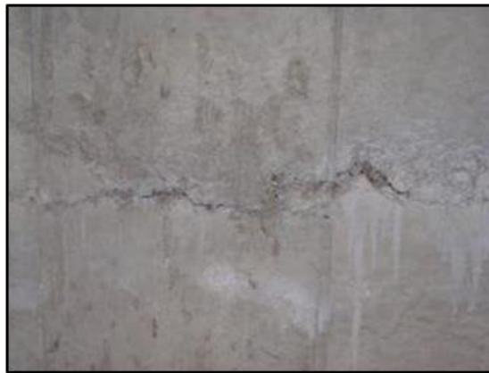
Figure 2.10. Crack-Like Formation Due to the Lack of Mixing of Two Batches of Concrete during the Pour (19).
