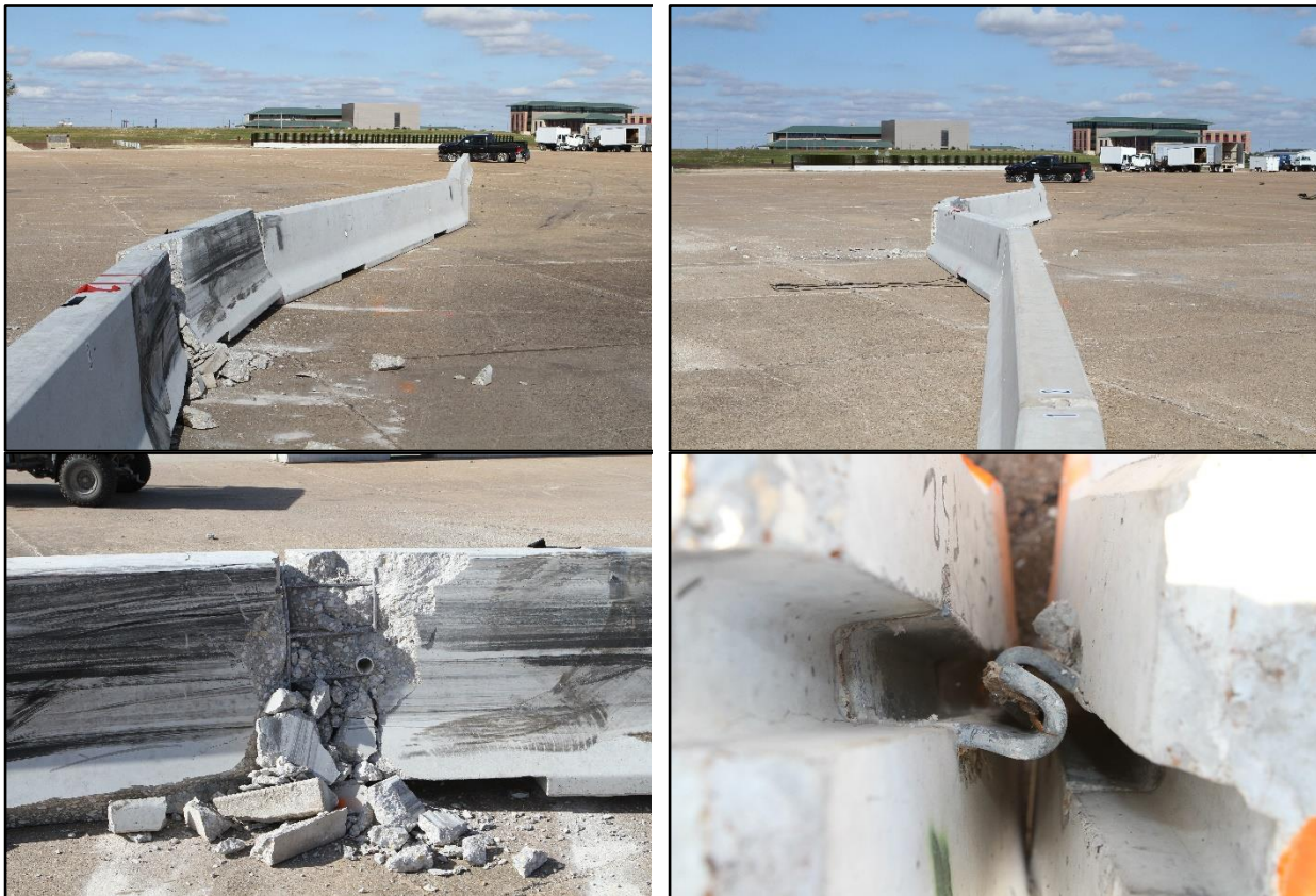
Figure 8.7. Damaged Portable Concrete Barrier after Test No. 440592-1.
