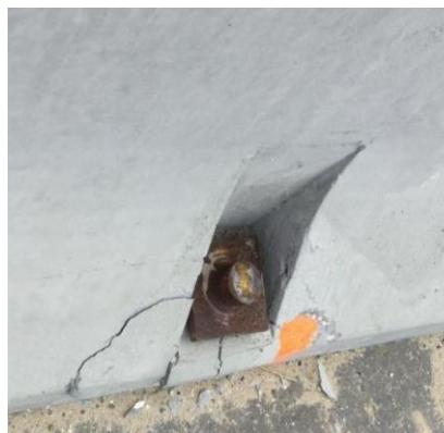
Figure 2.21. Example of Unacceptable Barrier with Broken Concrete at Anchor Slot Due to Shear Cracking— FDOT (31).
