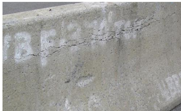
Figure 2.5. Clustered Horizontal Cracks Due to the Tight Clamping of Lifting Devices (10).
