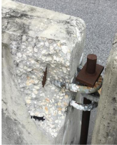
Figure 2.19. Example of Unacceptable Barrier with Connection Assembly Damage— FDOT (31).
