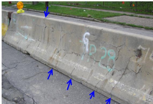
b. Unacceptable barrier
