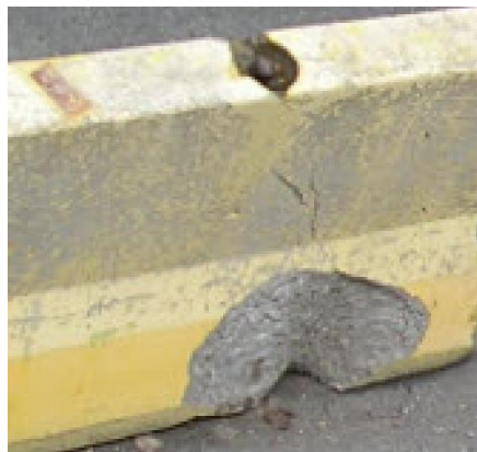
Figure 2.16. Unacceptable Barrier Due to Snag Risk—NYSDOT (27).
