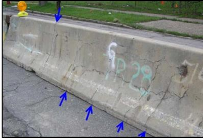
Figure 2.4. Cracking in Portable Concrete Barriers (8).
