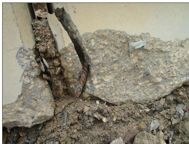
Figure 2.2. Corrosion of Reinforcing Bar Embedded in the Toe of the Concrete Barrier.
