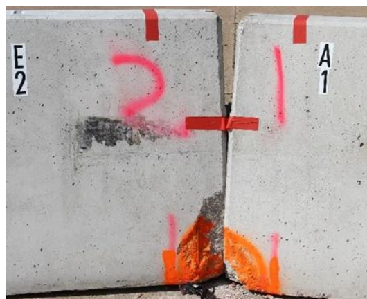
Figure 2.3. Spalling at the Toe of Barrier E Due to a Vehicle Crashing into the Joint between Barriers A and E.
