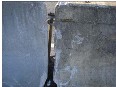
b. Unacceptable barrier
