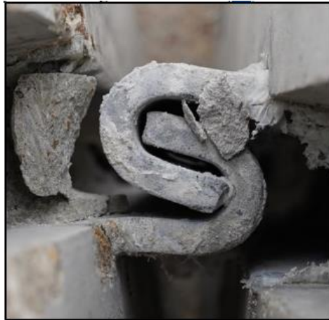
Figure 2.11. JJ Hook Connections: Top View of a JJ Hook Connection between Barrier Units.
