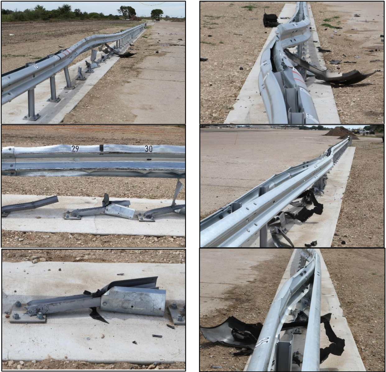
Figure 6.3. Surface-Mounted Median Guardrail after Test 440522-01-01.
