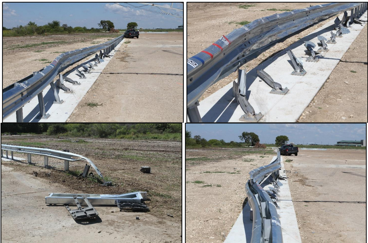
Figure 7.3. Surface-Mounted Median Guardrail after Test 440522-01-2.
