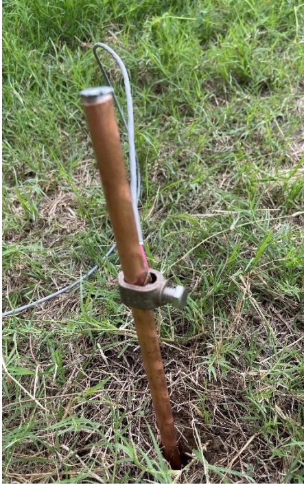
(a) Grounding Rod
