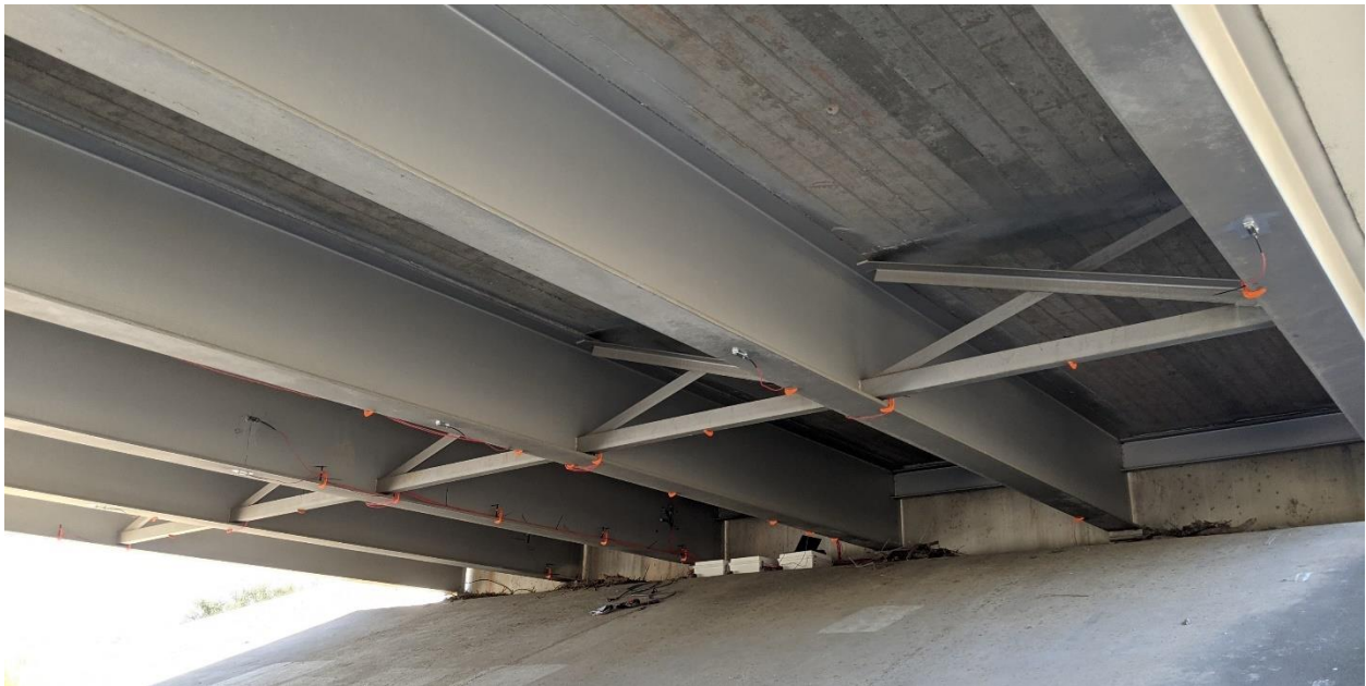
Figure 5.33. Midspan Strain Gauges (Bridge #3).
