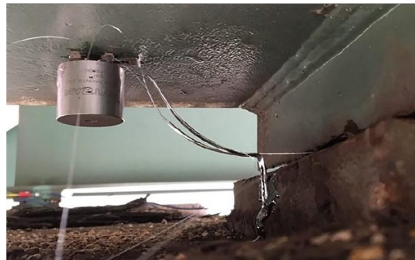
Figure 2.27. Installation Plan and Rotation Sensor Installed under the Girder (Oskoui et al. 2019).
