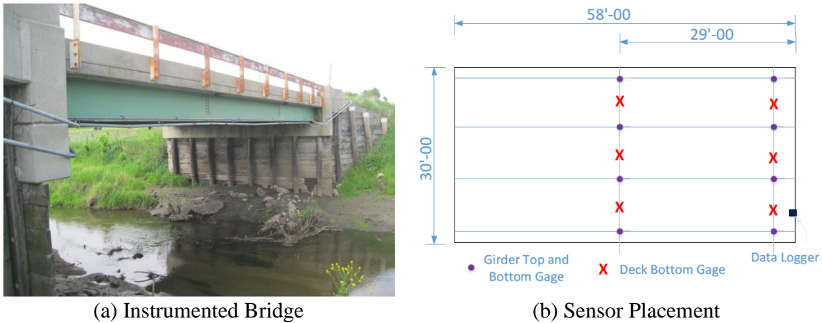
Figure 2.22. Instrumentation of the Bridge Located on Story County Road E-18 (Dahlberg et al. 2018).
