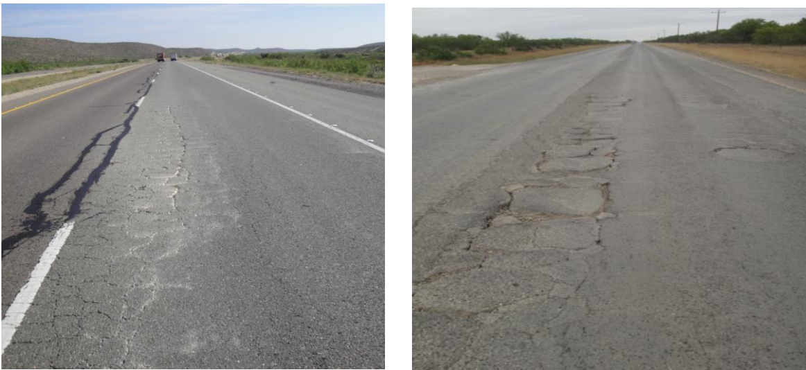
Figure 42. Early Severe Failures on Stiff CTB Layers with High Cement Contents.
