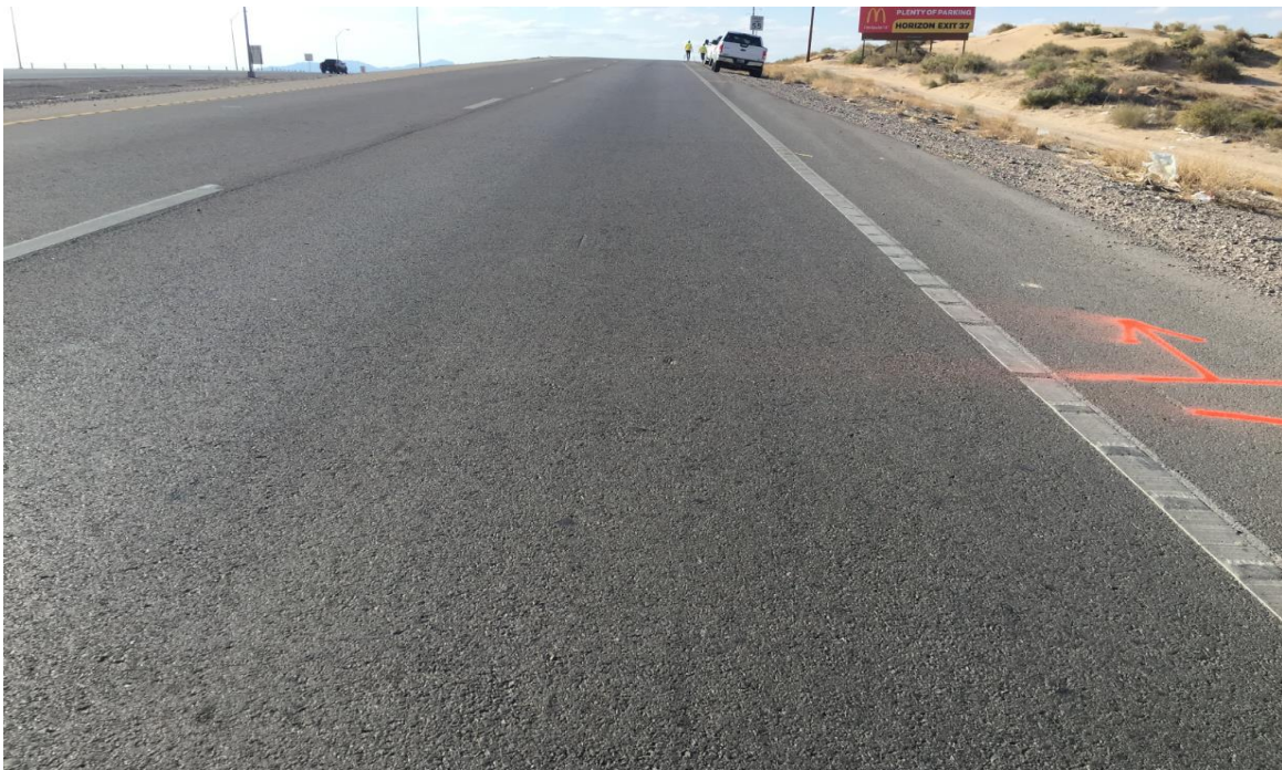
Figure 3-32. IH 10 Pavement Surface Condition in April 2021.
