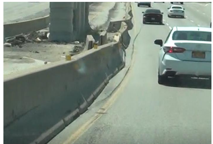
Figure 2. Barrier Deflection with Unanchored Temporary Barriers in Freeway Work Zones.
