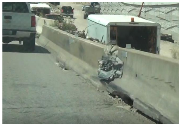
Figure 12. Example of a Barrier Connection between Damaged Barrier Segment Ends.
