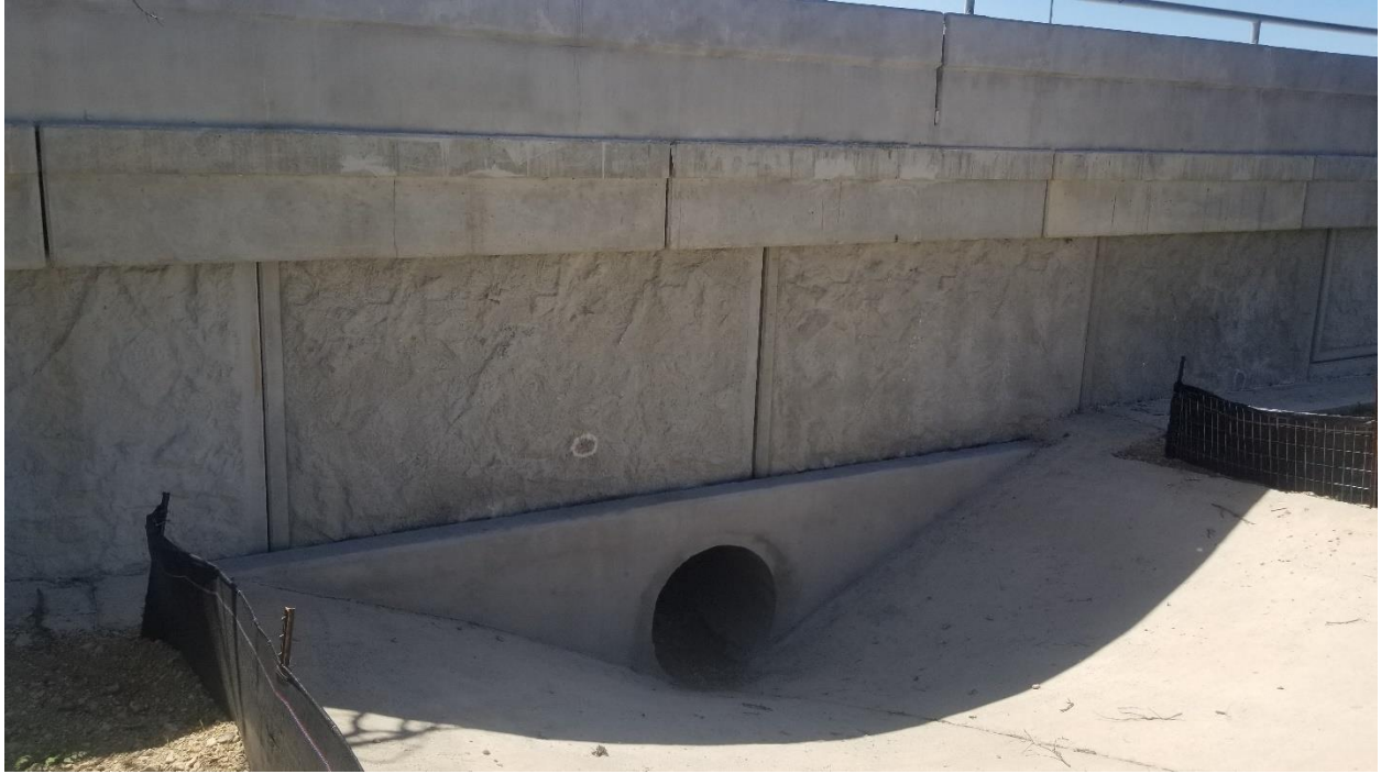
Figure 159. Drainage at Face of RWNB02.
