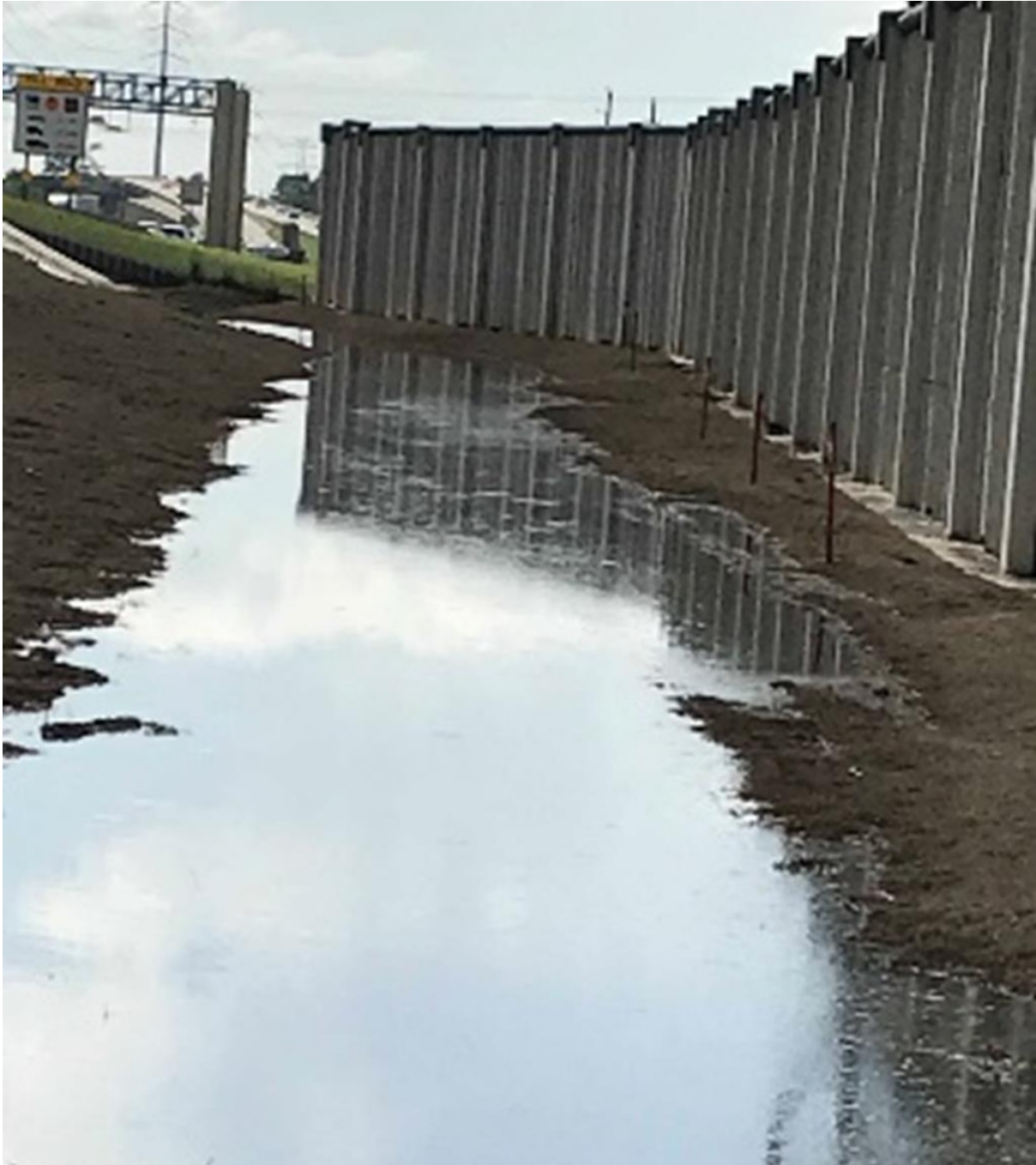
Figure 180. Drainage Issue near Noise Wall.
