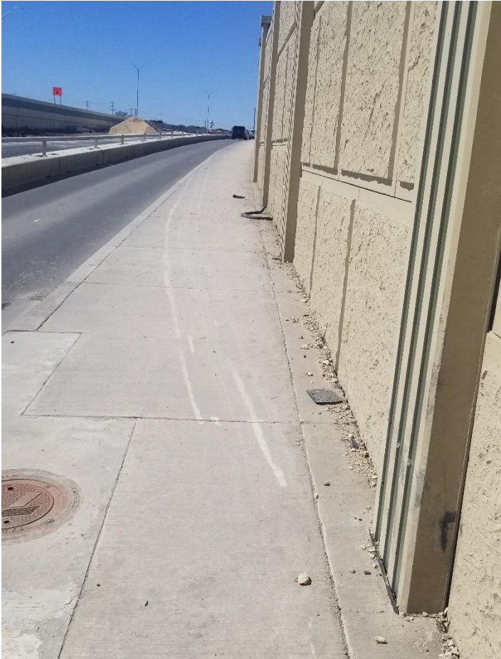
Figure 153. Visible Markings on SWNB04 and Sidewalk from Vehicle Strike.
