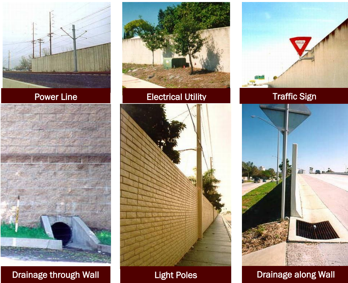
Figure 7. Interference between Walls and Drainage or Utilities (2).
