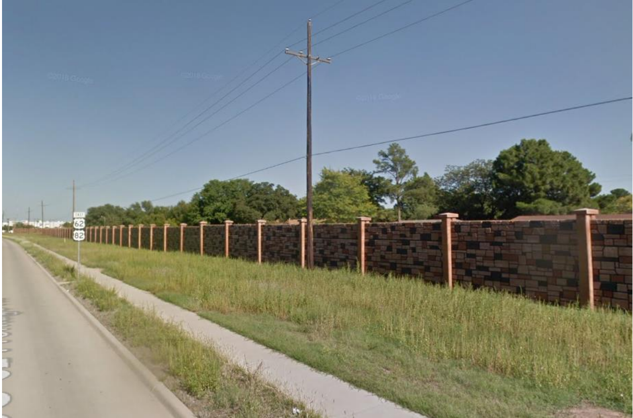
Figure 174. Noise Wall on Marsha Sharp Freeway in Lubbock, Freeway Side.
