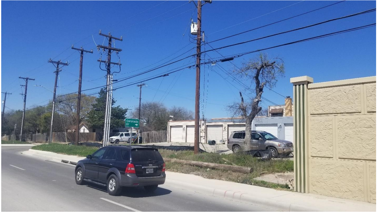
Figure 149. Omitted Portion of Wall at North End of SWNB04.
