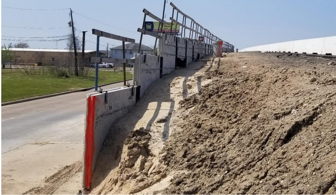
Figure 121. North-Facing View at Back of RW 12.
