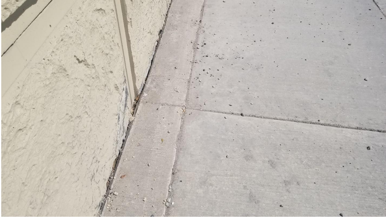
Figure 154. Visible Marking on SWNB04 from Vehicle Strike.
