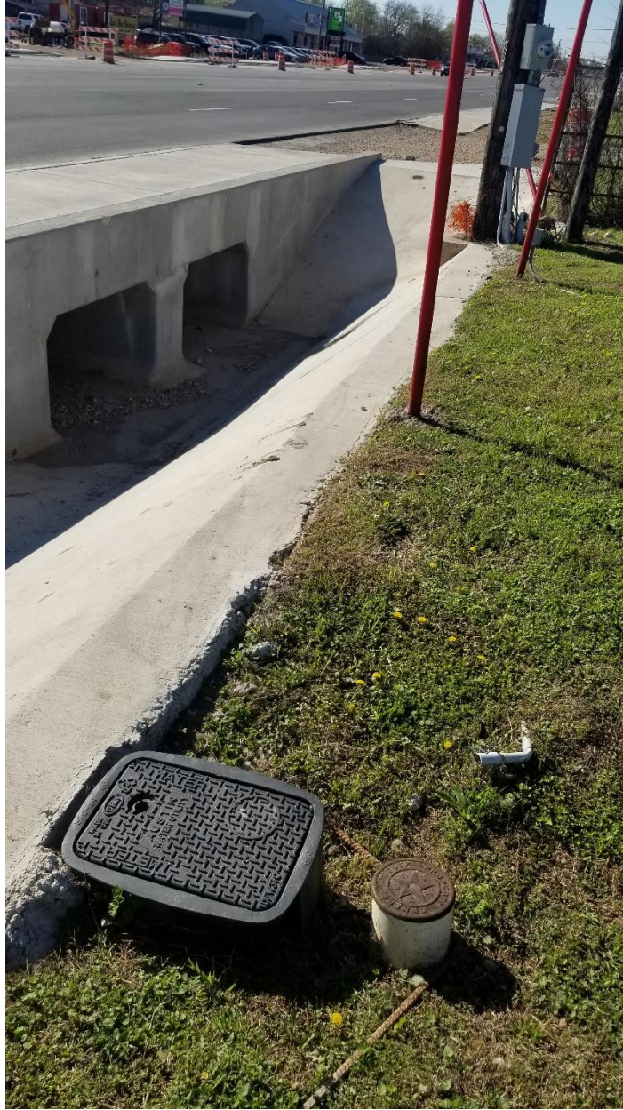
Figure 55. Water and Electrical Appurtenances near Southbound Headwall.
