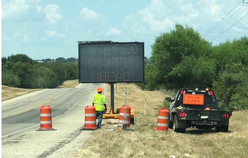
Figure 16. PCMS Displaying STOPPED TRAFFIC AHEAD Message.
