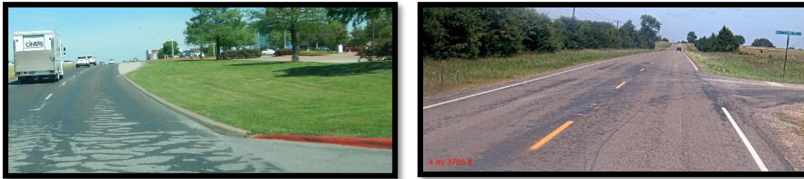
Figure 7. Damage at Intersections.
