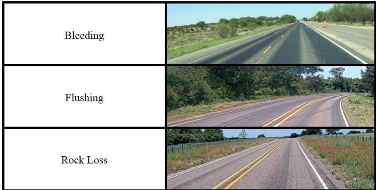
Figure 2. Seal Coat Defects.
