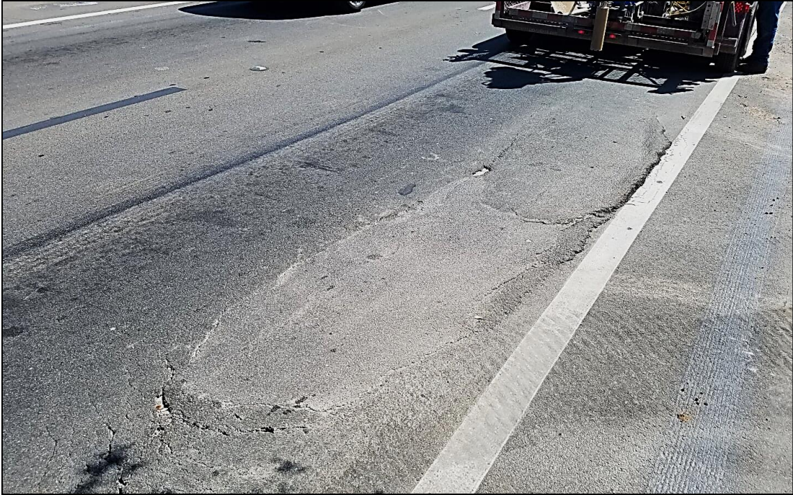
Figure 28. Eastbound Outside Lane at Cherry Street.
