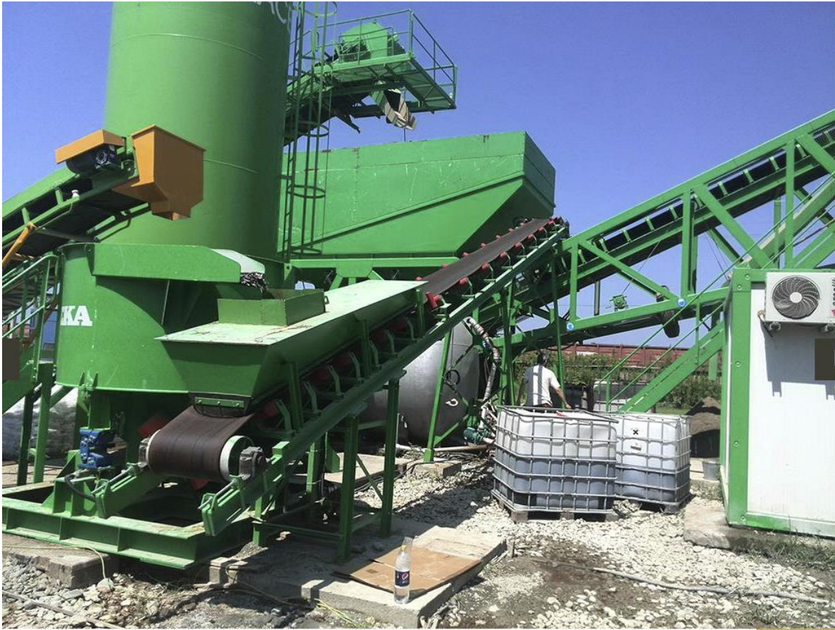
Figure 2.6. Example of Automated Fiber Dosing System at Plant (Berkshire Engineering Supplier 2022).
