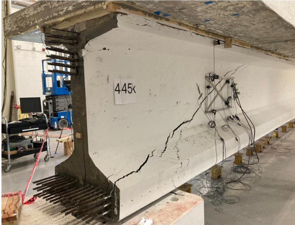
Figure 6.55. Tx54 Shear Test 2: Shear Span of Unreinforced End at Failure.
