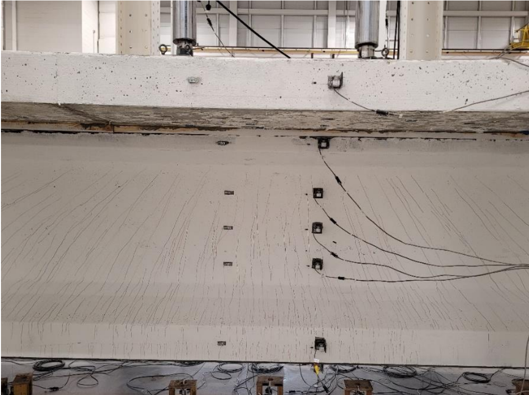
Figure 5.33. Cracks in Constant Bending Moment Region Tx54.
