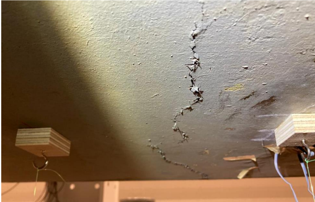
Figure 5.25. Fibers Bridging the Crack at the Underside of the Soffit of Tx34-2.
