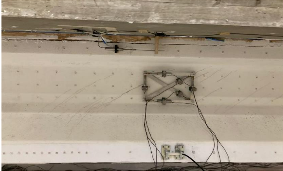
Figure 5.16. Tx34-1 Shear Cracks at Unreinforced End at 450 Kips.
