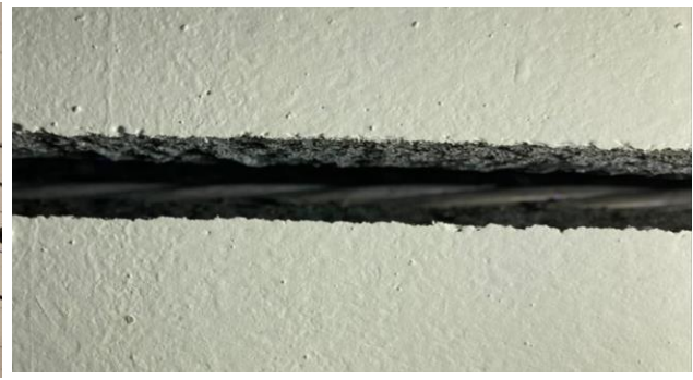
(c) Exposed Prestressing Strand
