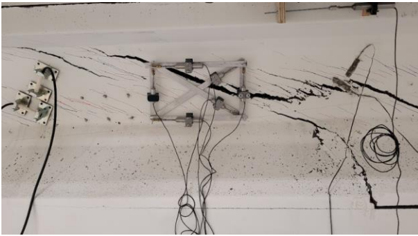
(a) Photograph of Tx34-2 at Peak Load
