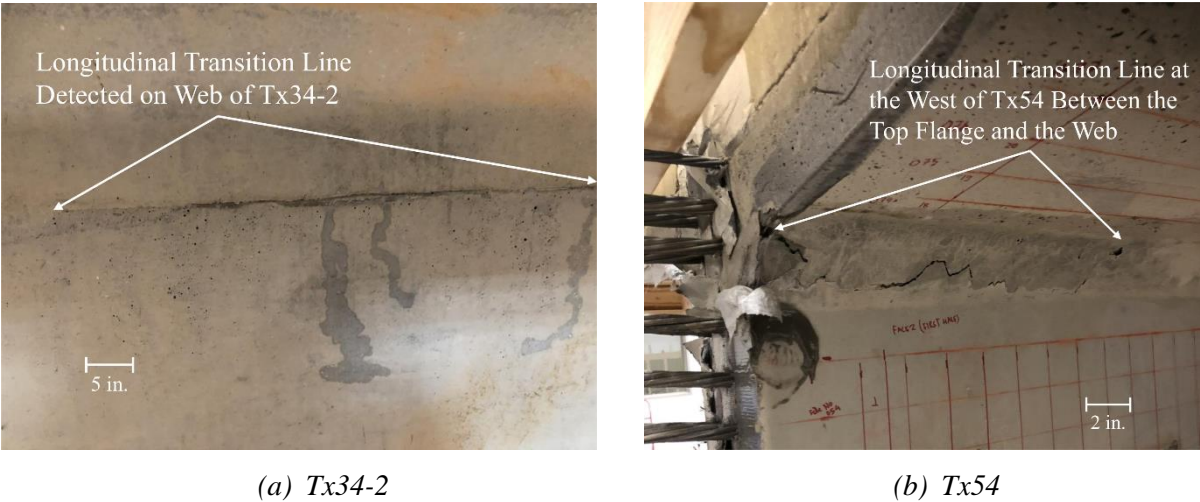
Figure 7.28. Longitudinal Transition Line Detected on the Web.
