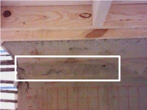
(c) FLIR Digital Image—South-west
