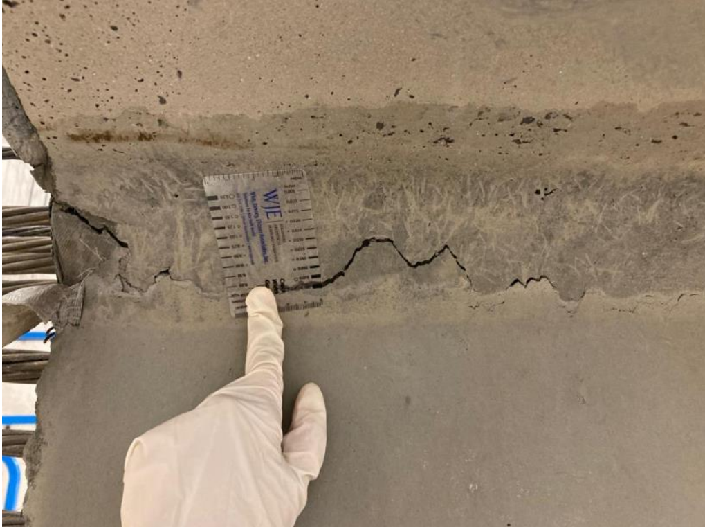
Figure 6.27. Crack Opening at Transition Line Tx54.
