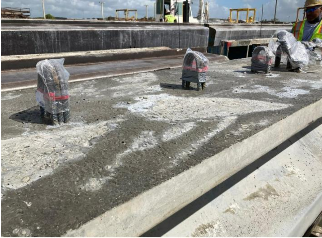
Figure 6.17. Tx34-2 Top Girder Surface without Any Surface Preparation.
