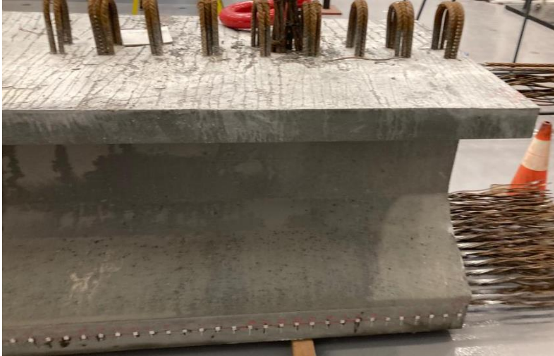
Figure 6.11. Tx34-1 Top Girder Surface Grooved for Roughness.
