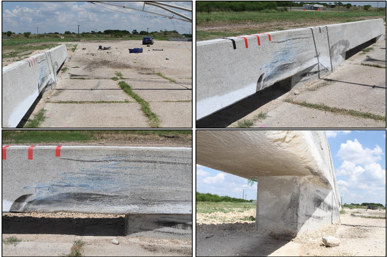
Figure 9.3. TxDOT LSMB after Test No. 469760-06-1.
