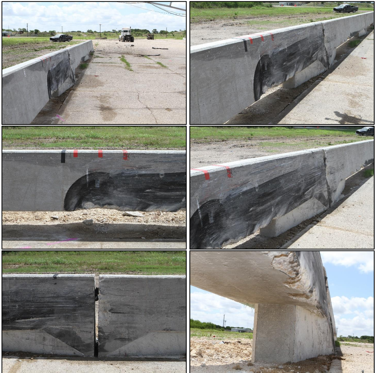
Figure 10.3. TxDOT LSMB after Test No. 469760-06-2.
