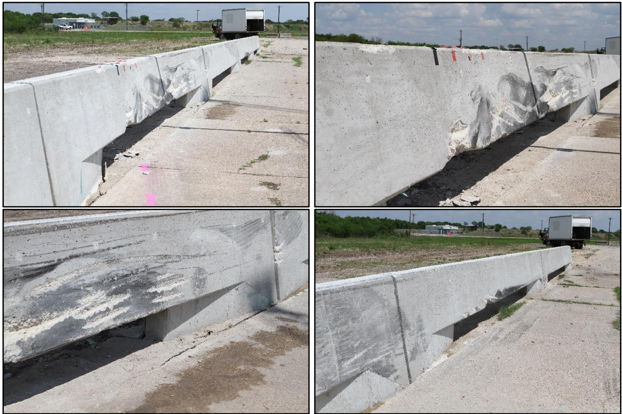
Figure 11.3. TxDOT LSMB after Test No. 469760-06-3.
