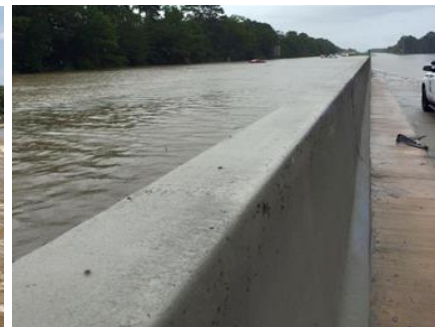
(b) The flooded westbound lanes of Interstate 12 with a concrete barrier damming up the flow of water (Louisiana) (3).
