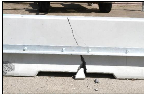
Figure 2.20. Concrete Crack after MASH Test 3-11 (Retrofit System).
