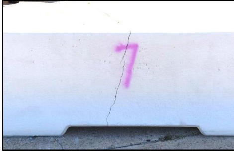
Figure 2.19. Concrete Crack after MASH Test 2-11.
