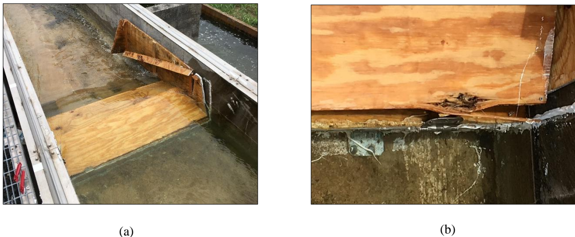
Figure 5.8. (a) Weir Barrier Failure; (b) Hinged Connection Failure.
