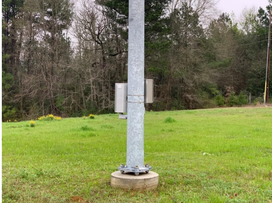
Figure 37. Equipment Integrated at the Intersection.
