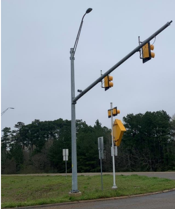
a. Mast Arm with Sensor.
