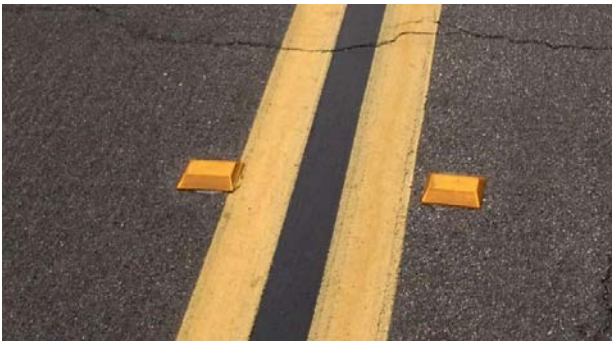
(a) Surface-mounted RRPMs.
