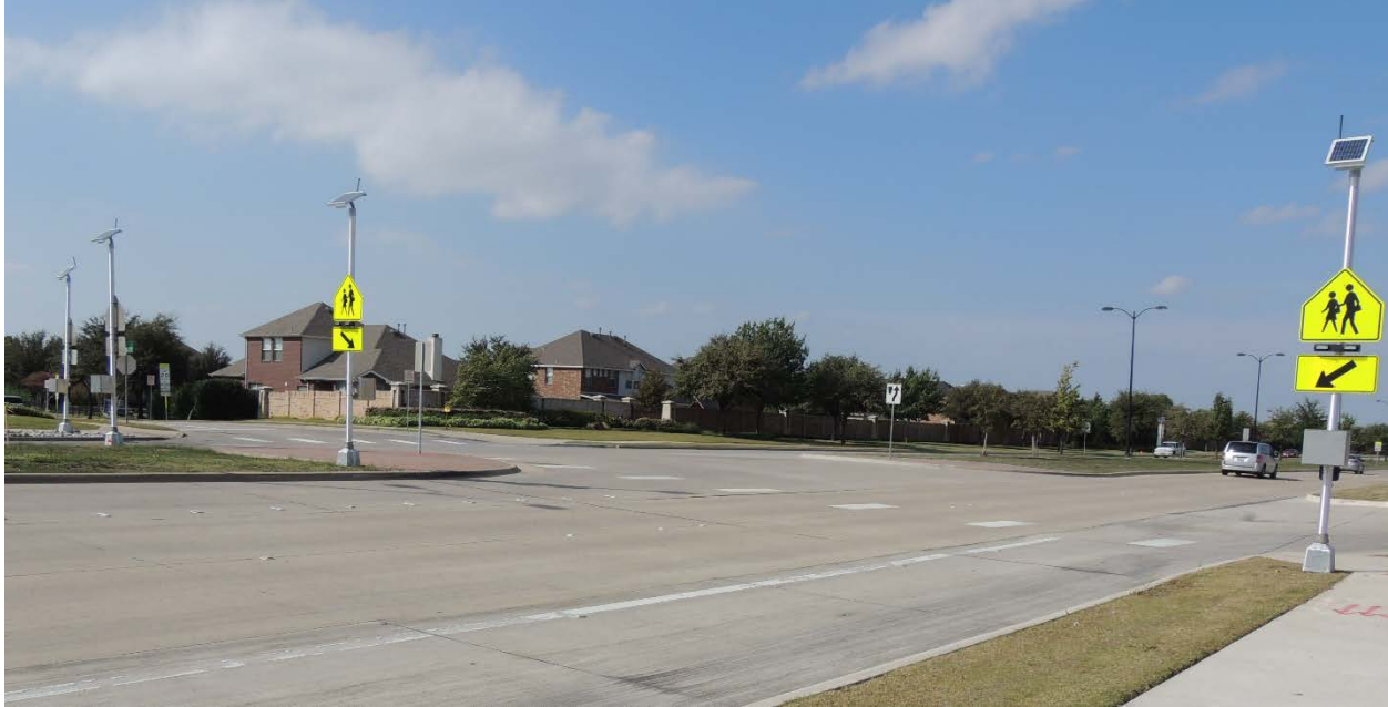
Figure 12. RRFB Installed on Roadside at School Crossing on 45-mph Roadway.
