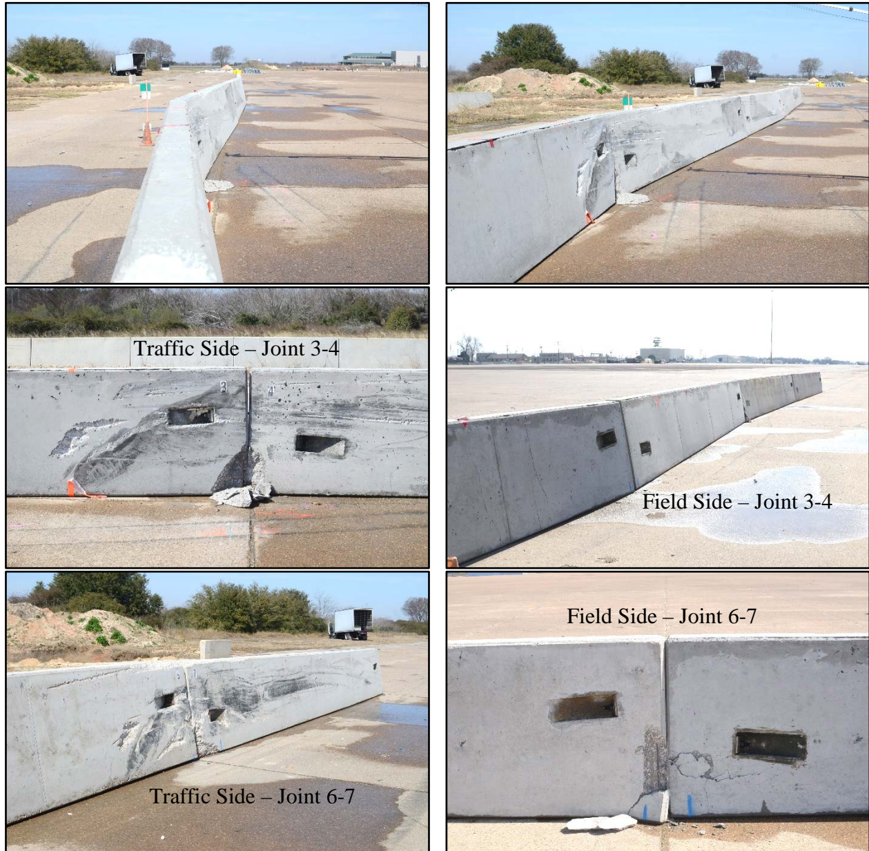
Figure 5.3. Barrier after Test No. 469688-3-1.
