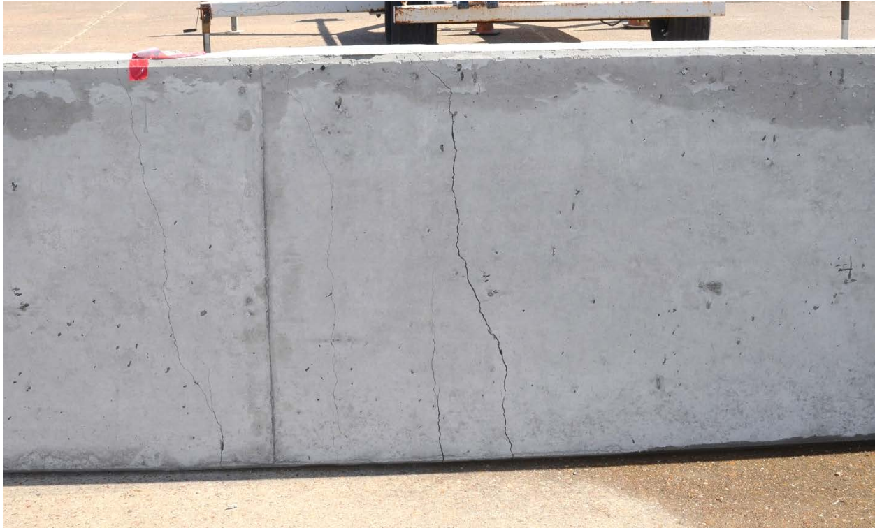
Figure 5.4. Traffic Side of Segment 4 after Test No. 469688-3-1.
