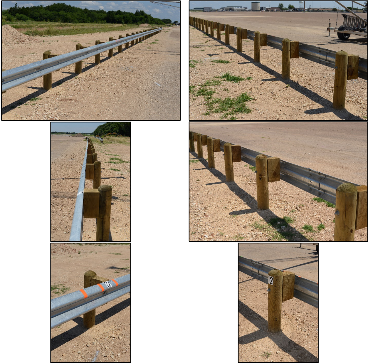
Figure 2.2. Modified TxDOT Round Wood Post Guardrail System prior to Testing.
