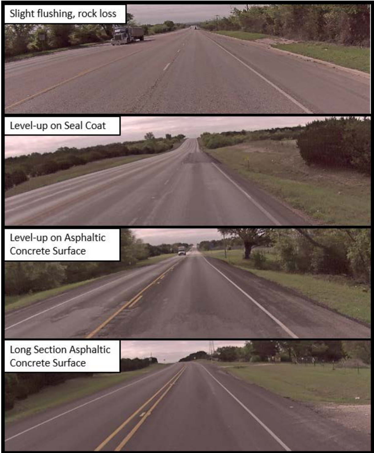
Figure 35. SH 36, Waco District, Surface Conditions.
