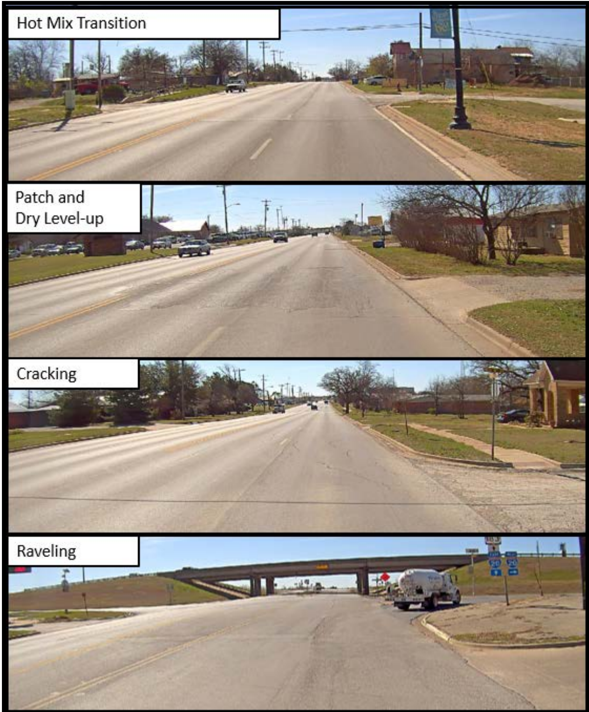
Figure 28. US 183 Surface Conditions.
