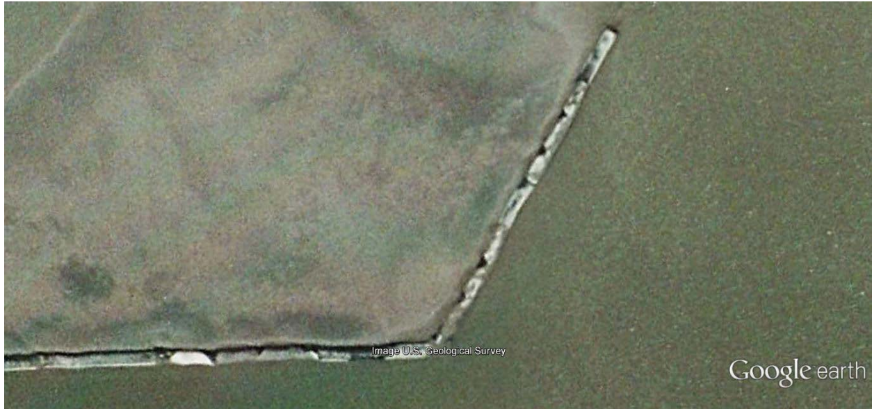
Figure 13. Close-Up of Geotextile Tubes after a Few Years of Performance in January 2004.
