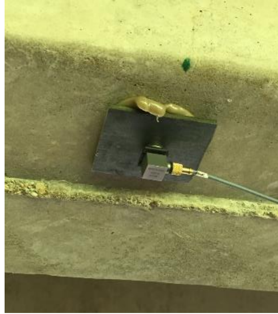
(b) Installed Accelerometer
