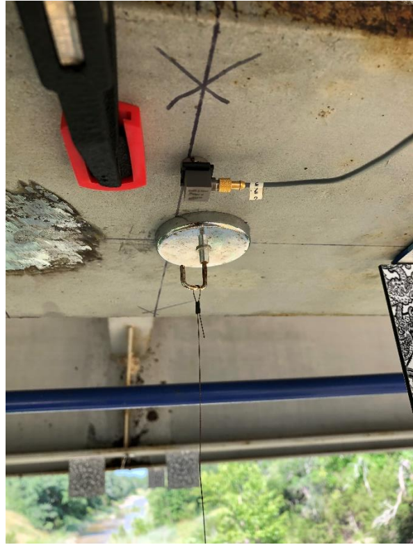
(b) Example of Installed Accelerometer
