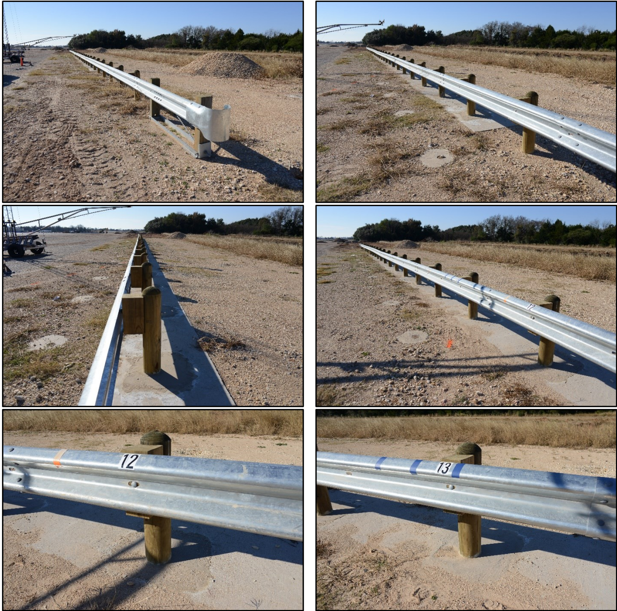
Figure 12.2. Round Wood Post Guardrail in a Concrete Mow Strip prior to Testing.
