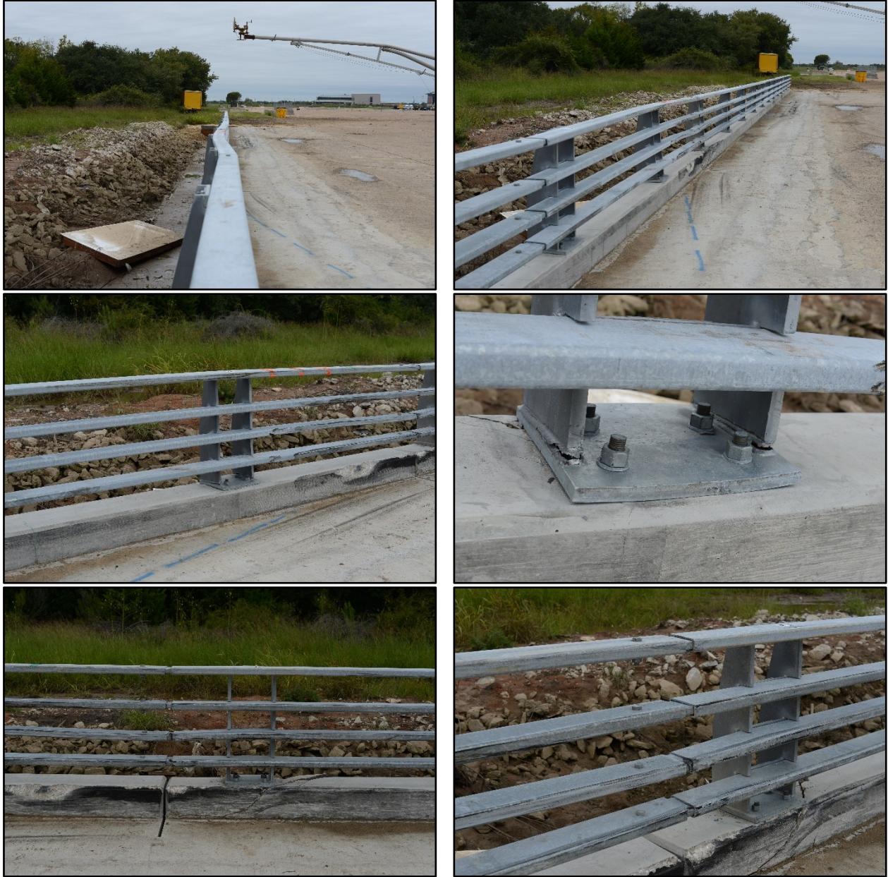
Figure 2.5. C1W Bridge Rail after Test No. 469469-1.
