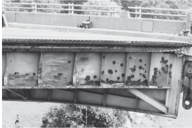
Figure 2.2. Collapse of the Mianus River Bridge (Fisher 1997).
