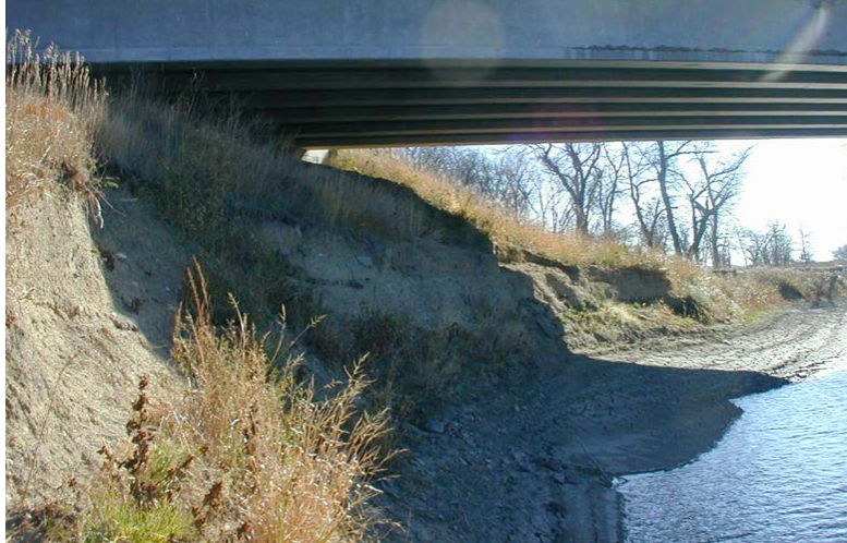
Figure 20. Scour at the Left Abutment of SR 37 over James River during the Flood.
