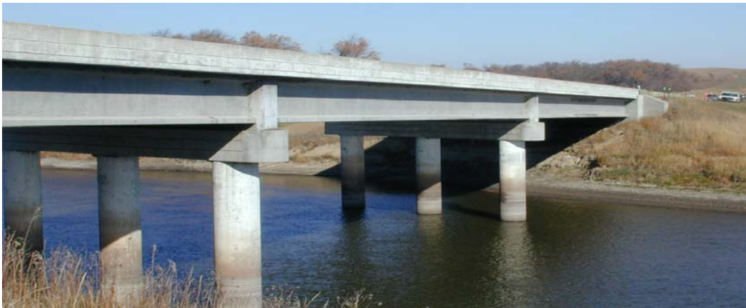
Figure 18. SR 37 over James River after the Flood—Looking at the Left Abutment from the Downstream.
