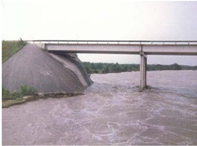
Figure 29. Right Abutment Failure at US 90 over Nueces River.
