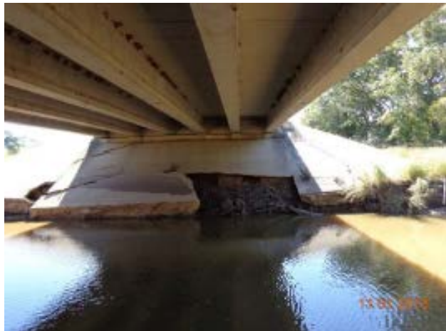
Figure 24. Damaged Concrete Riprap at the Right Abutment of FM 937 over Montgomery Creek.
