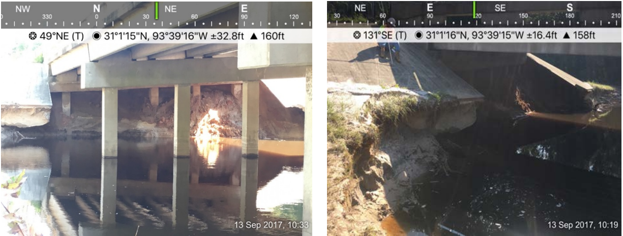
Figure 21. Left Abutment Failure at FM 692 over McGraw Creek.
