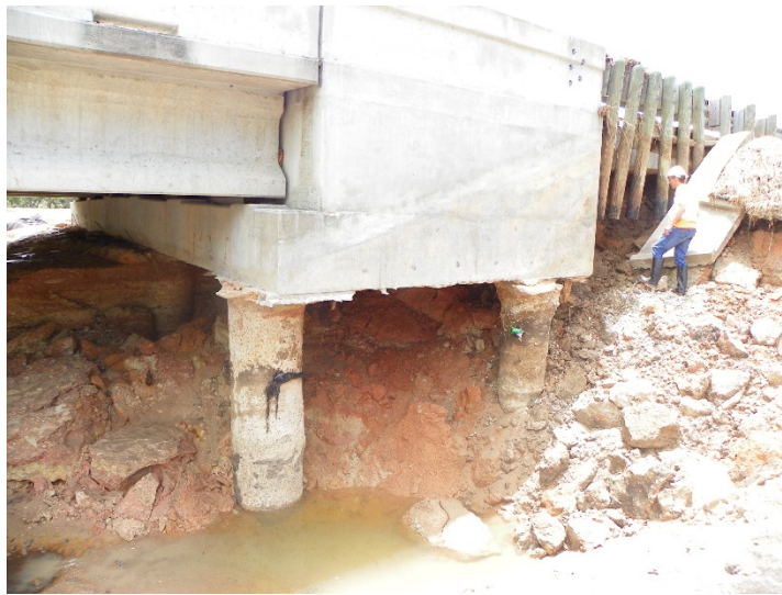
Figure 28. Right Abutment Failure at SH 105 over Rocky Creek.
