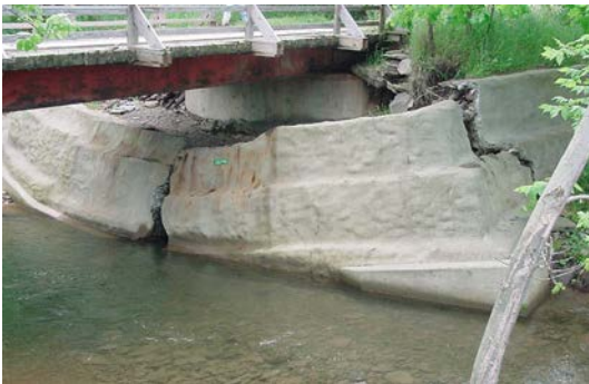
Figure 32. Abutment Foundation Failure by Vertical Loading.
