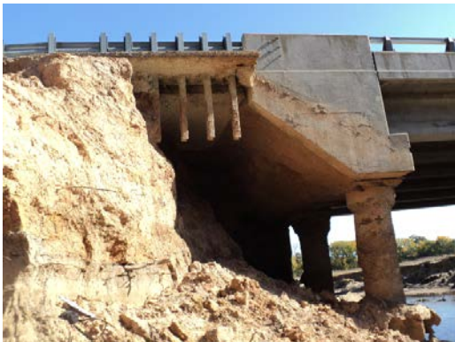
Figure 34. Slope Stability Failure of the Abutment Embankment.
