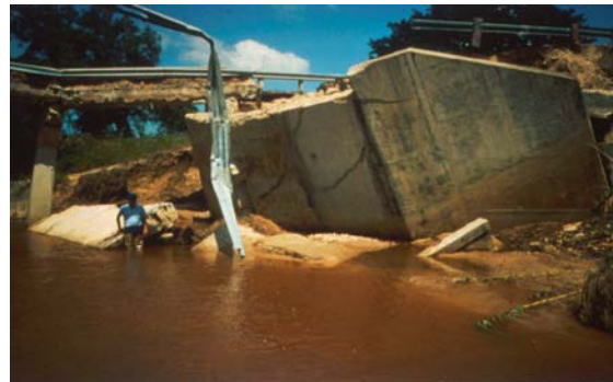
Figure 33. Abutment Foundation Failure by Horizontal Loading.
