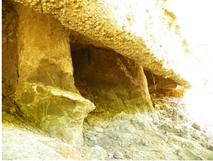
Figure 26. Voids under the Left Abutment Concrete Riprap of CR 309 over Rocky Creek.
