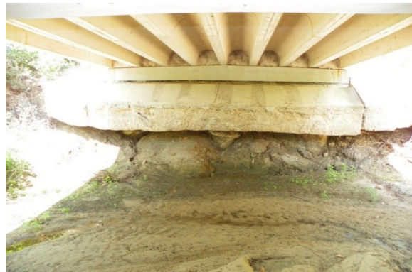
Figure 35. Erosion of the Embankment Soil.
