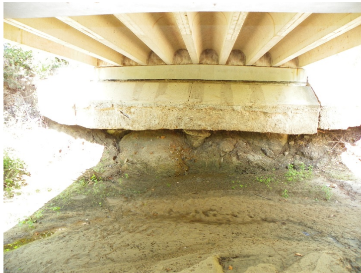
Figure 25. Scour at the Left Abutment of CR 309 over Rocky Creek.
