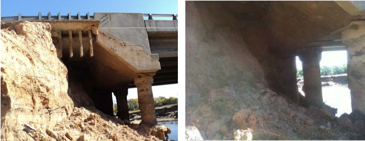
Figure 23. Left Abutment Failure at FM 937 over Montgomery Creek.
