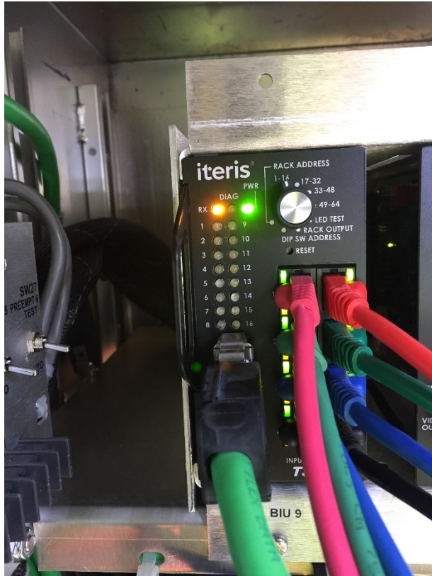
Figure 47. Iteris TS-2 IM Module Installed in the Cabinet.
