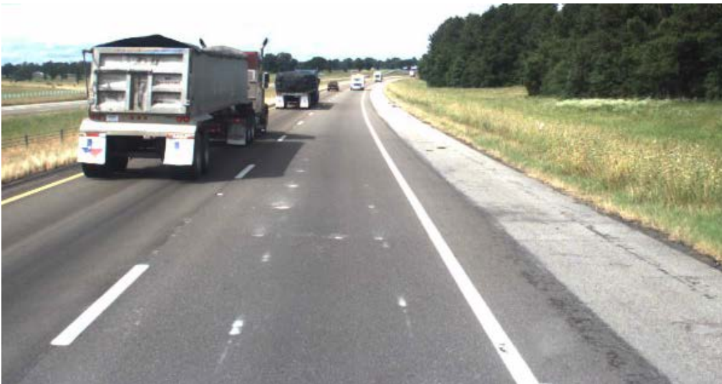
Figure 105. IH 30 Westbound Location with Deep Rutting and Potential Striping.
