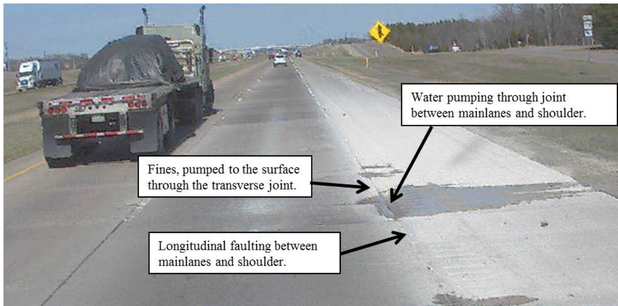
Figure 71. Water Pumping through Pavement and Shoulder Faulting at Project Site.
