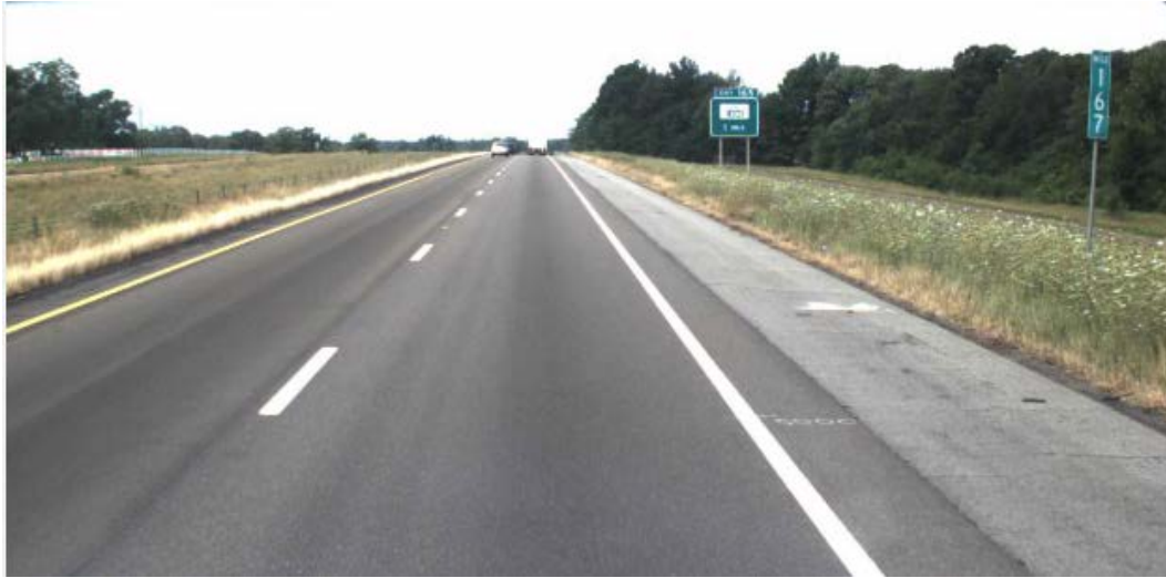
Figure 104. IH 30 Westbound Area with Deep Rutting.
