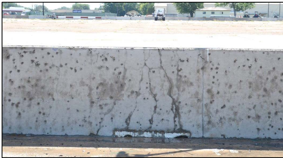
Figure 5.42. Field Side-Center of Barrier after Test No. 468957-B9.
