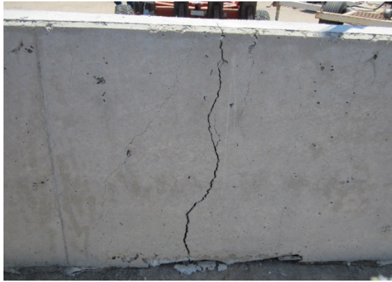
(a) CR10FGnet crack pattern
