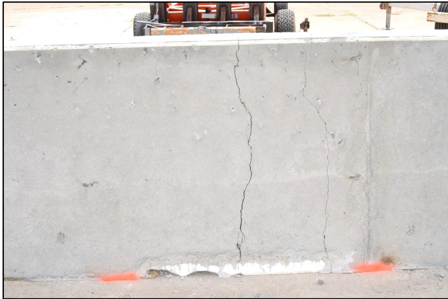
Figure 5.33. Field Side-Center of Barrier after Test No. 468957-B8.
