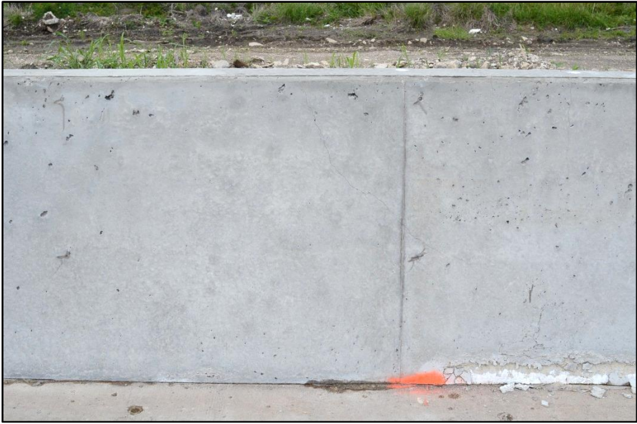
Figure 5.31. Traffic Face of Barrier after Test No. 468957-B8.
