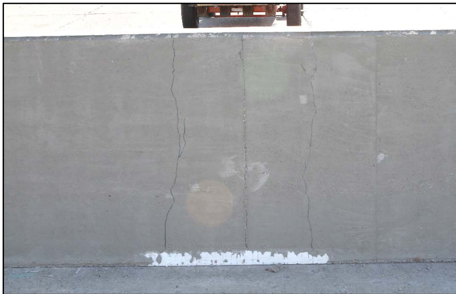
Figure 5.7. Field Side-Center of Barrier after Test No. 468957-B4.
