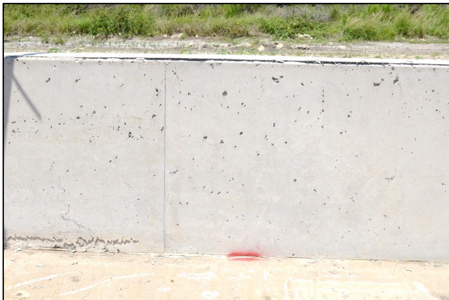
Figure 5.49. Traffic Face of Barrier after Test No. 468957-B10.
