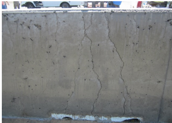
(e) PR5FCR5F crack pattern
