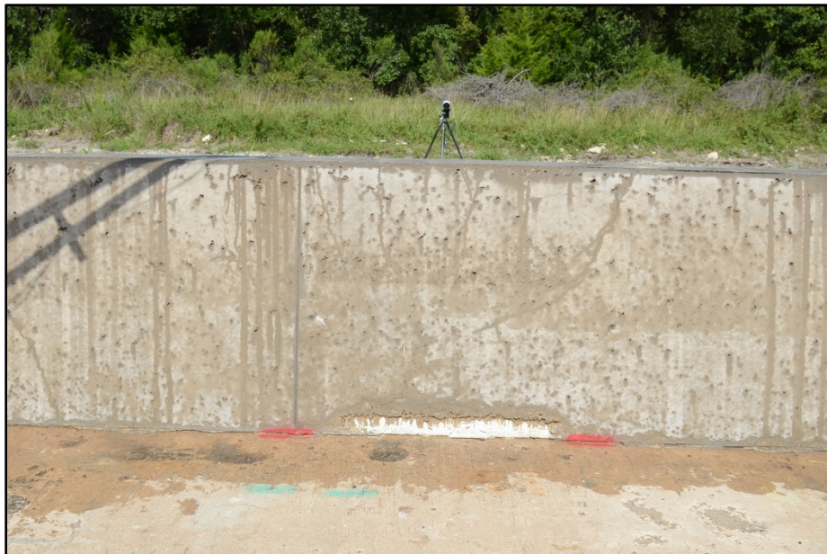
Figure 5.40. Traffic Face of Barrier after Test No. 468957-B9.
