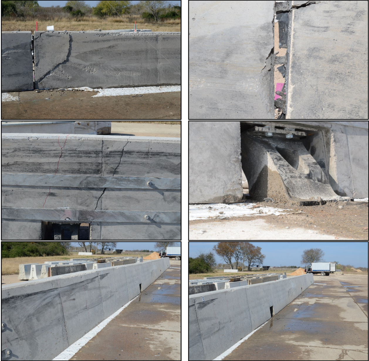
Figure 11.5. Damage to Barrier #3 after Test No. 468958-3.
