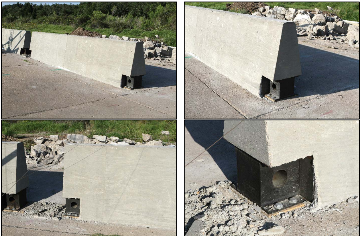
Figure 5.1. Single-Slope Median Barrier with Shear Fender Anchor Plate before Test No. 468957-B4.
