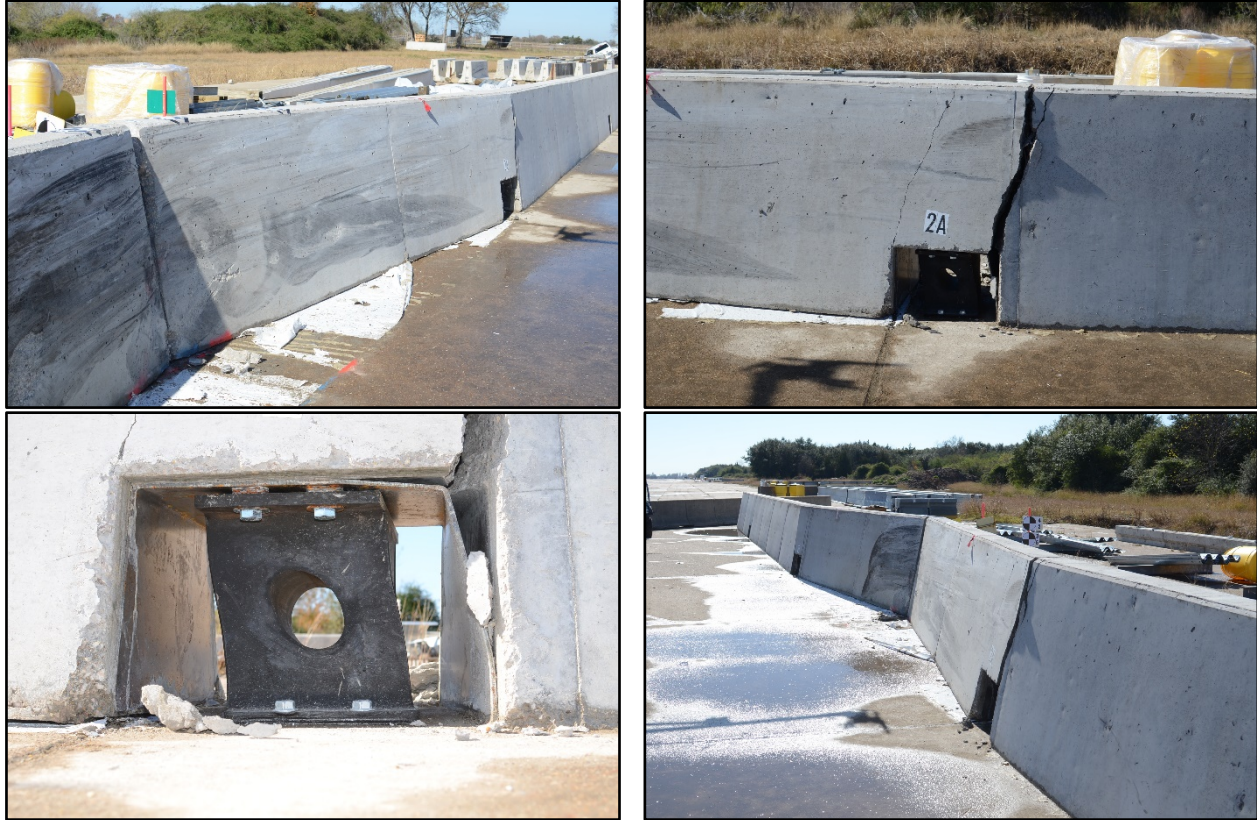
Figure 10.5. Damage to Barrier #2 after Test No. 468958-2.
