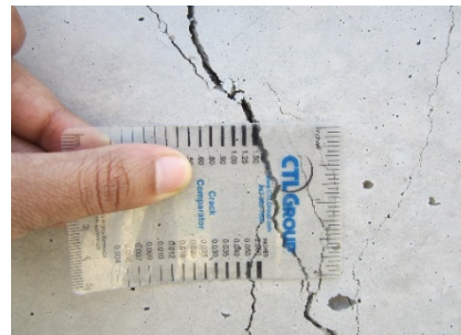
(f) PR5FCR5F maximum crack width measurement
