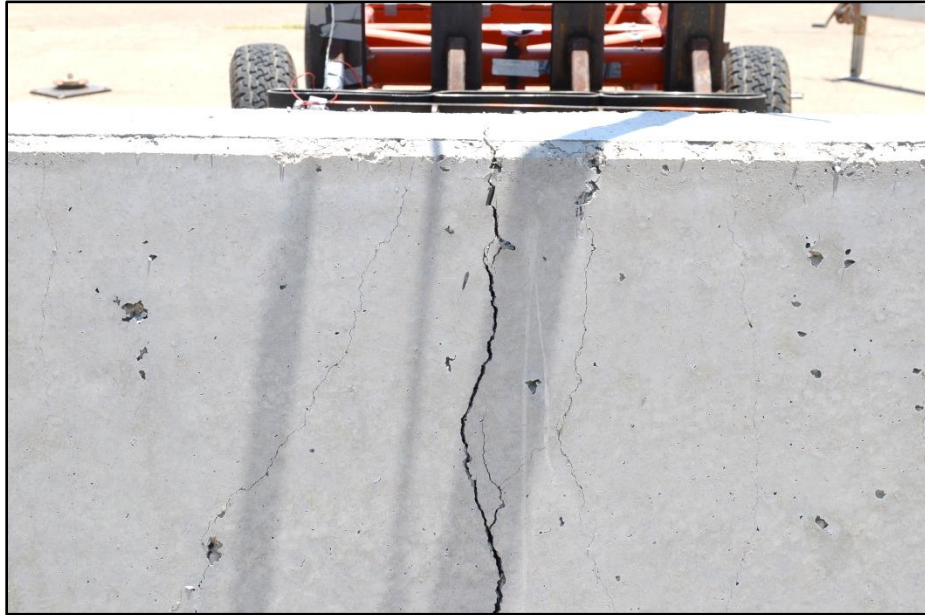
Figure 5.50. Top of Barrier after Test No. 468957-B10.
