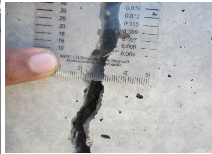
(b) CR10FGnet maximum crack width measurement
