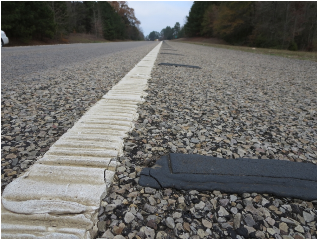
Figure 12. SH 8 Edge Line Inverted Profile Marking with Audible, and Shoulder Rumble Bars.
