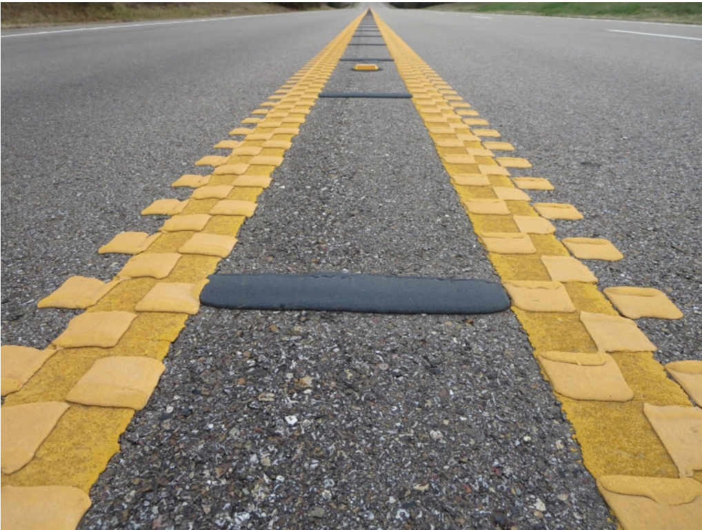
Figure 14. US 259 Checkerboard Pattern Audible Marking with Rumble Bars.
