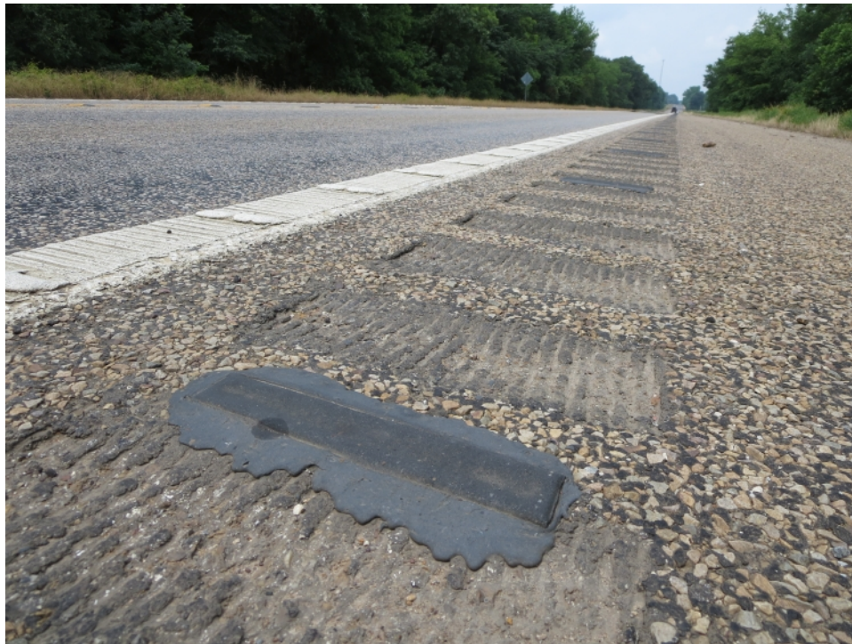
Figure 8. US 79 Edge Line Inverted Profile Marking with Audible, Milled Rumble Strips, and Rumble Bars.
