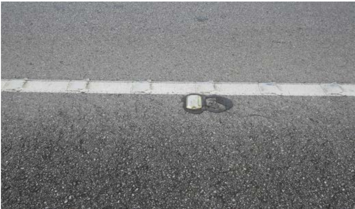
Figure 15. Aged Profile Pavement Marking near Bastrop.
