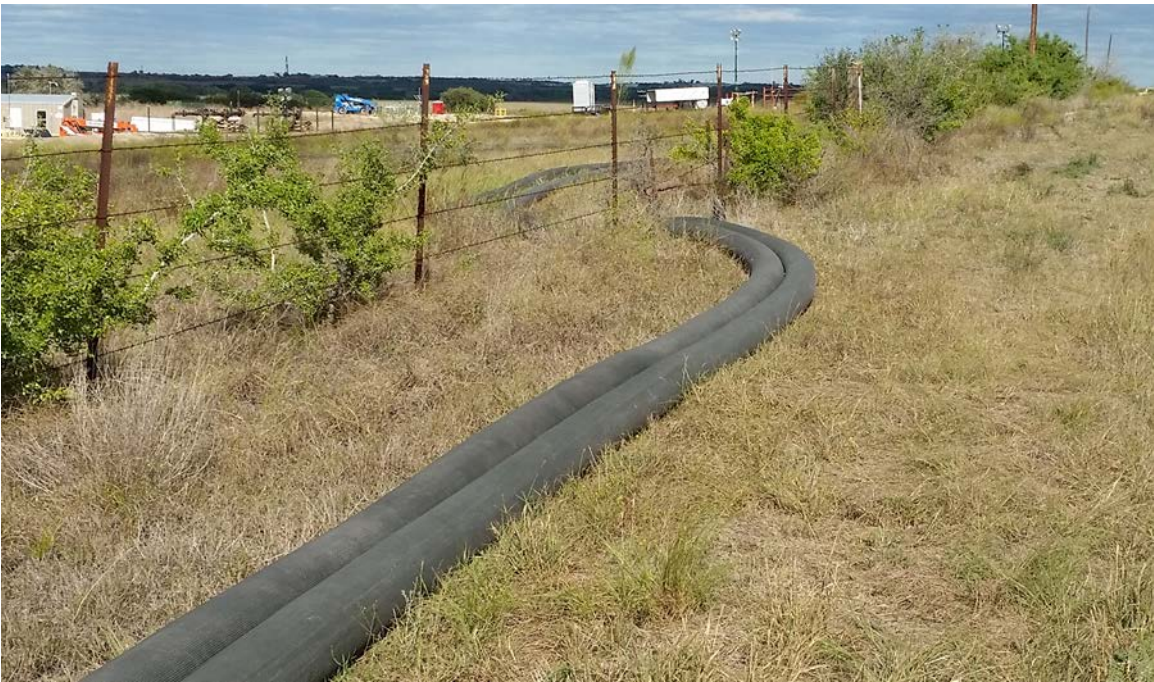
Figure 24. Temporary Pipelines Crossing Right-of-Way Line without Signage.
