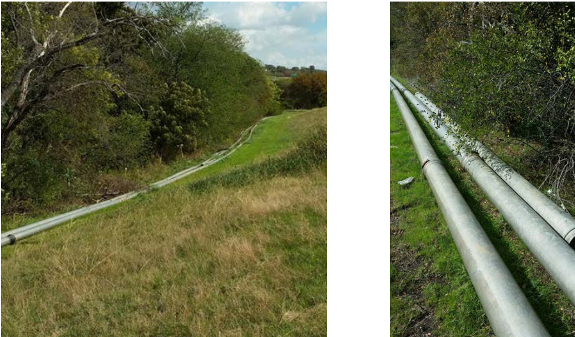
Figure 13. Temporary Aluminum Pipeline in the Barnett Shale Region.
