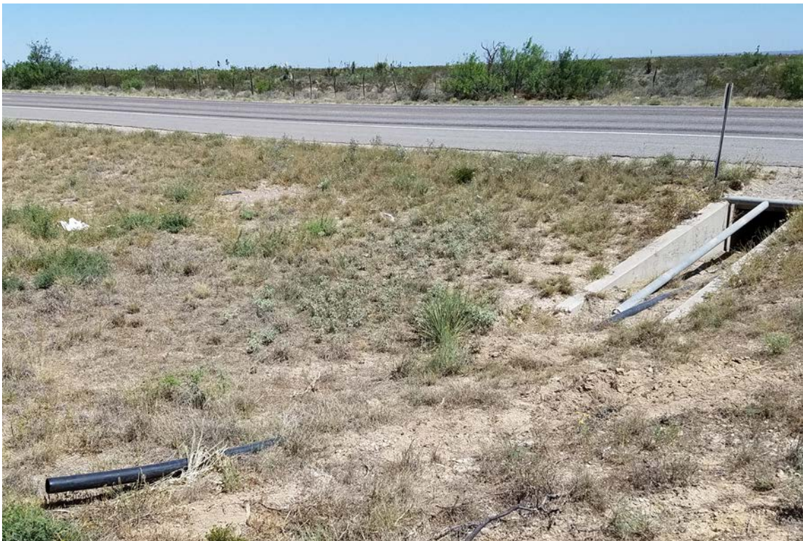
Figure 21. Temporary Pipeline Cut and Left in Place in a Culvert.
