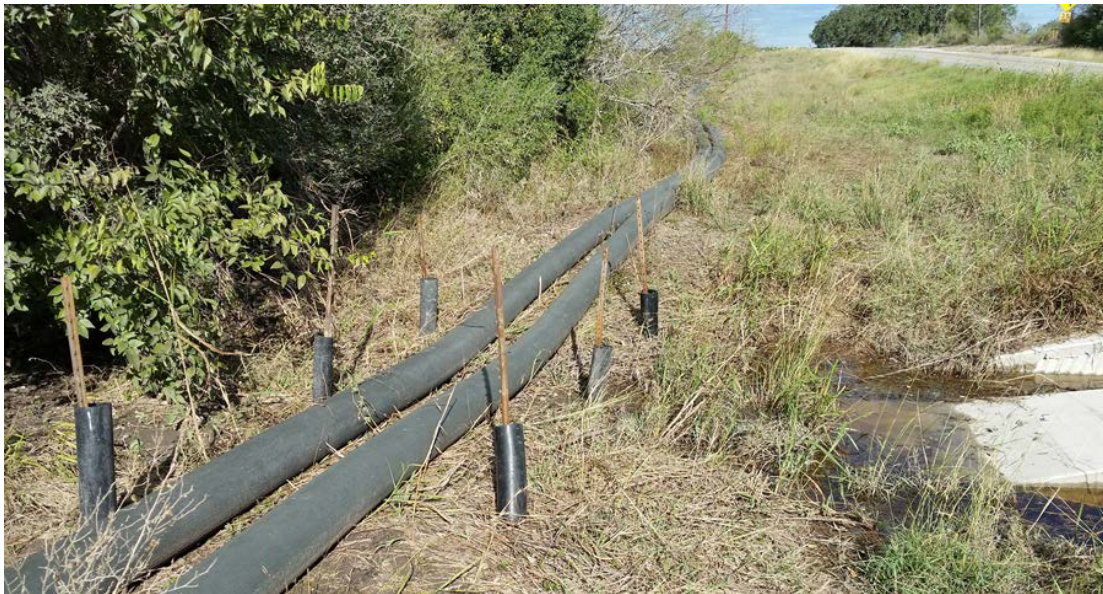
Figure 16. Metal Fence Posts Used to Anchor a Temporary Pipeline in a Drainage Location.
