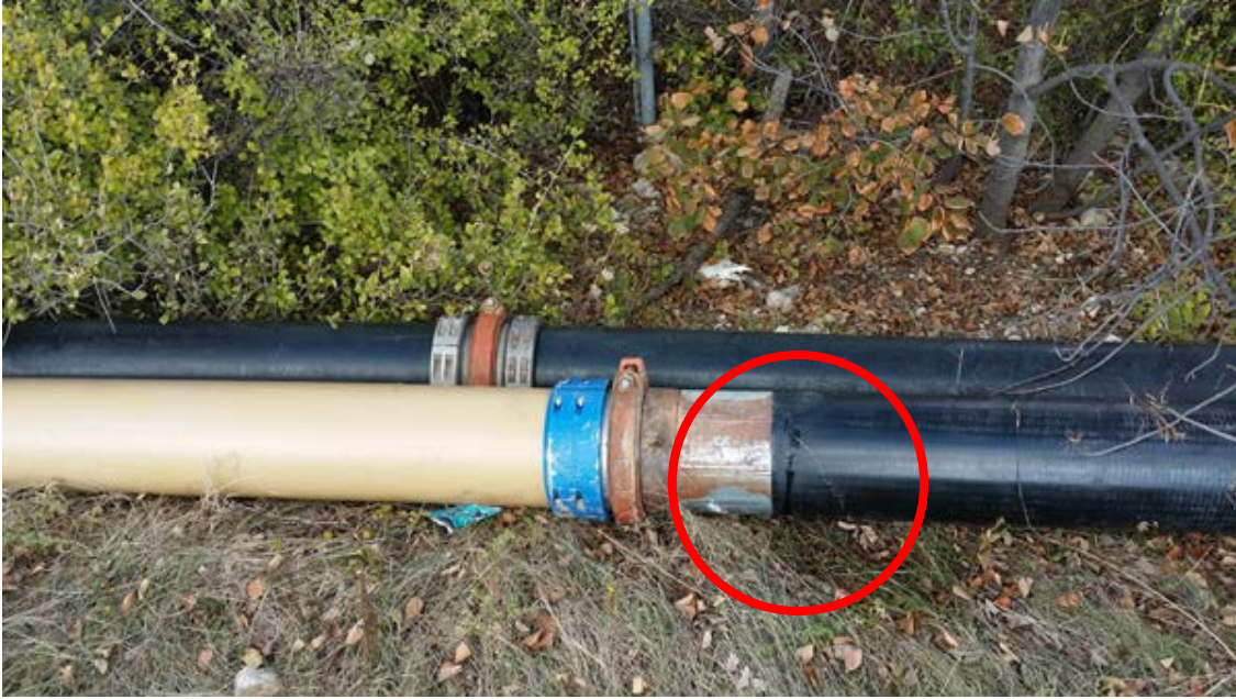
Figure 19. Temporary Pipeline Small Pinhole Leak.
