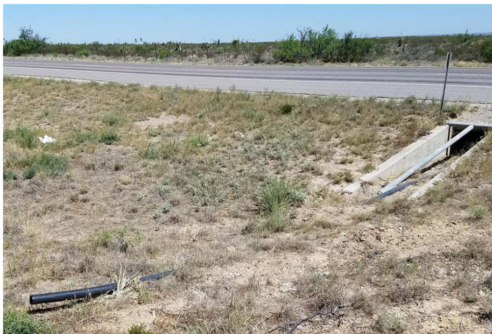
Figure 4. Temporary Pipeline Cut and Abandoned in a Highway Culvert.
