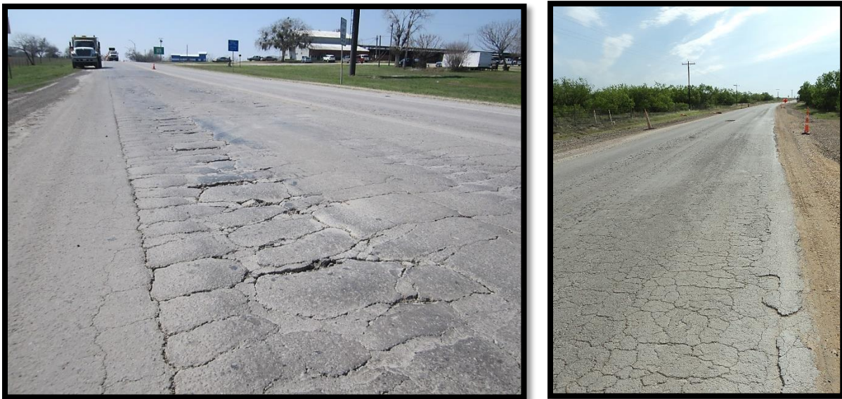
Figure 1. Energy-Sector Pavements in Need of Rehab.
