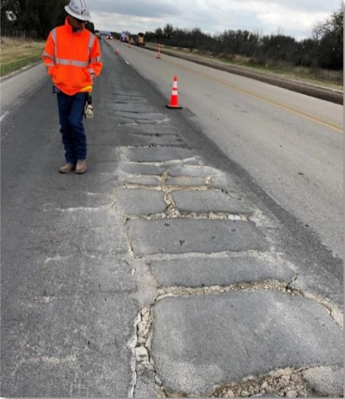
Before FDR (photo courtesy TxDOT)
