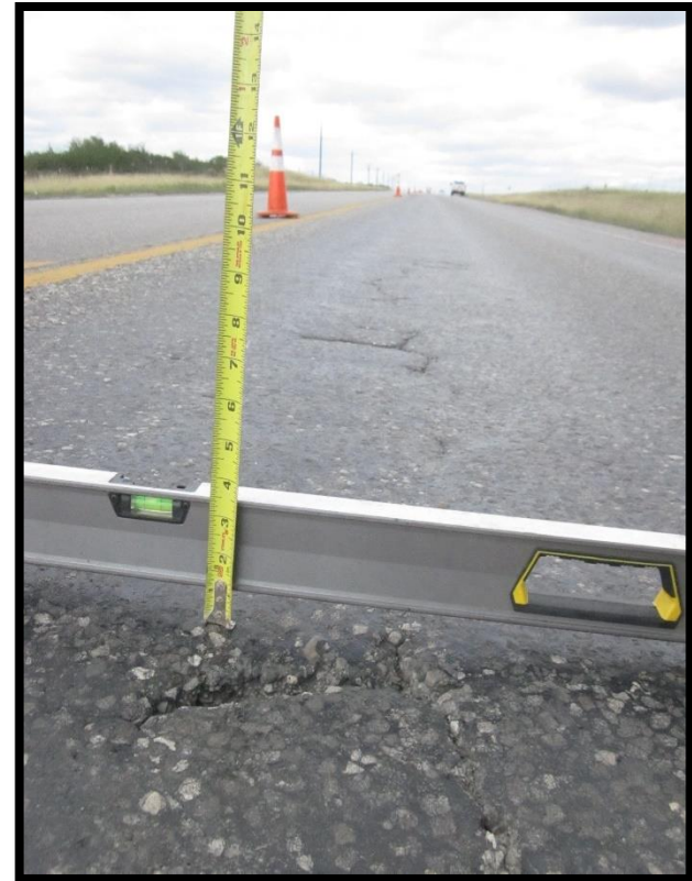
Wide, deep rutting suggests triaxial failure
