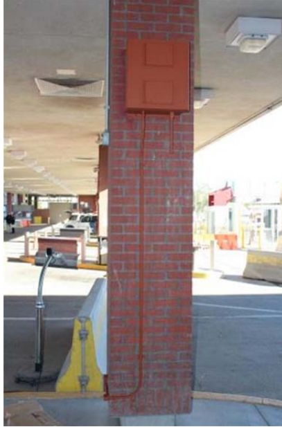
Figure 32. Bluetooth Reader Installed at CBP’s Primary Inspection Facility at the Ysleta-Zaragoza POE.
