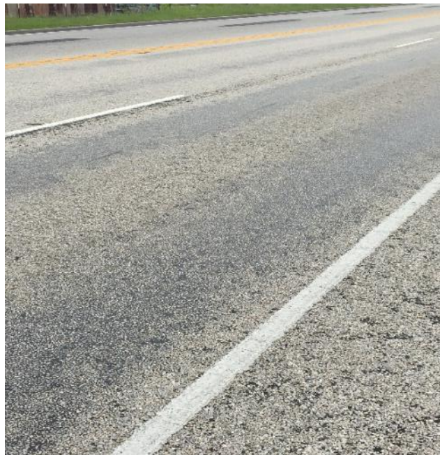
b. Surface Condition of Pavement Section B
