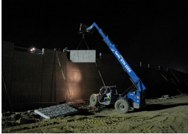
Figure 14. Placement of Precast Concrete for Mechanically Stabilized Earth Wall in Fort Worth.
