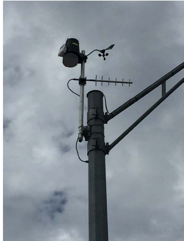
Weather Monitoring Station
