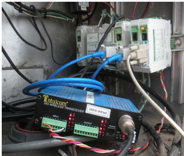
Figure 50. Image of Contact Closures and Radio.
