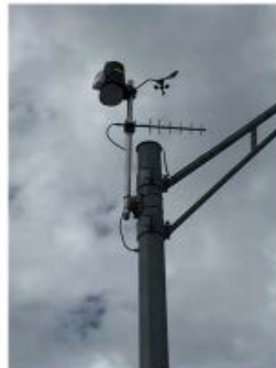
Weather Monitoring Station
