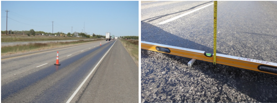
Figure 8. High Surface Rutting in IH35 Cotulla.
