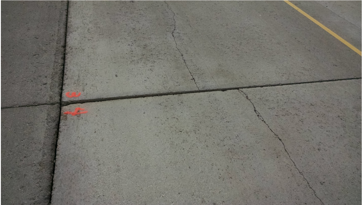
Figure 145. Location 3 and 4 (Joint Separation and Faulting).
