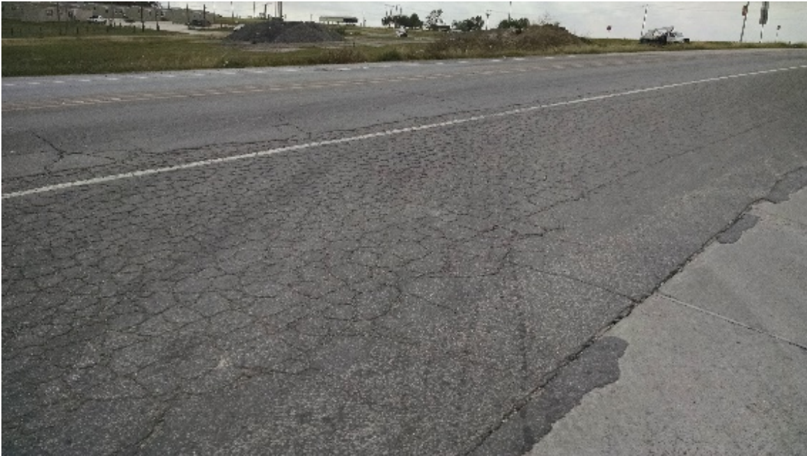
Figure 111. Alligator Cracking Distress Located on SH 123, Approach Lane toward US 181.
