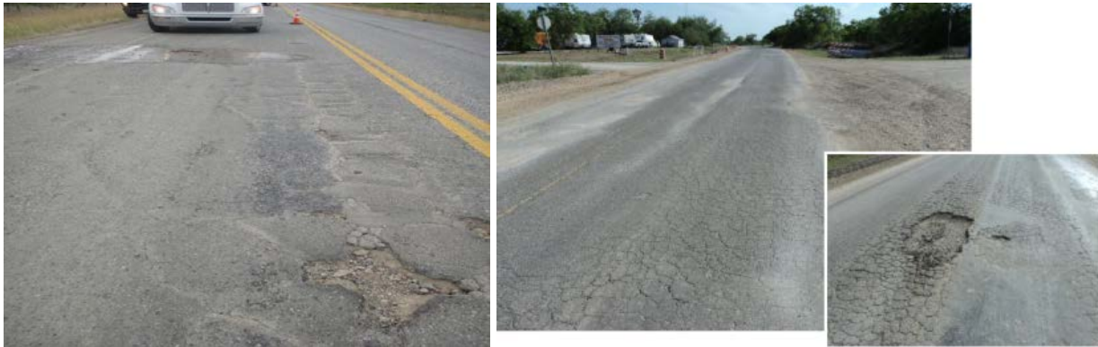
Figure 1. Pavement Damage Caused by Overload Trucks in Energy Development Areas.
