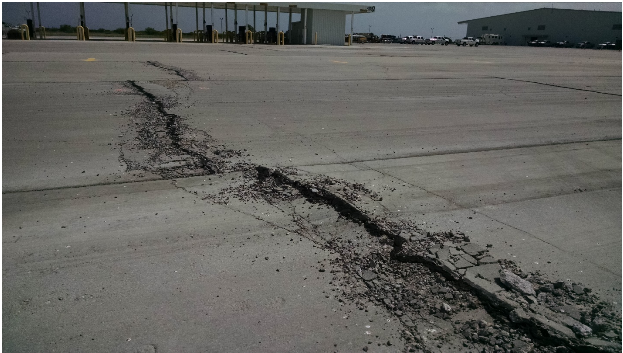
Figure 147. Major Blow-Up Located in the Center of the Property.
