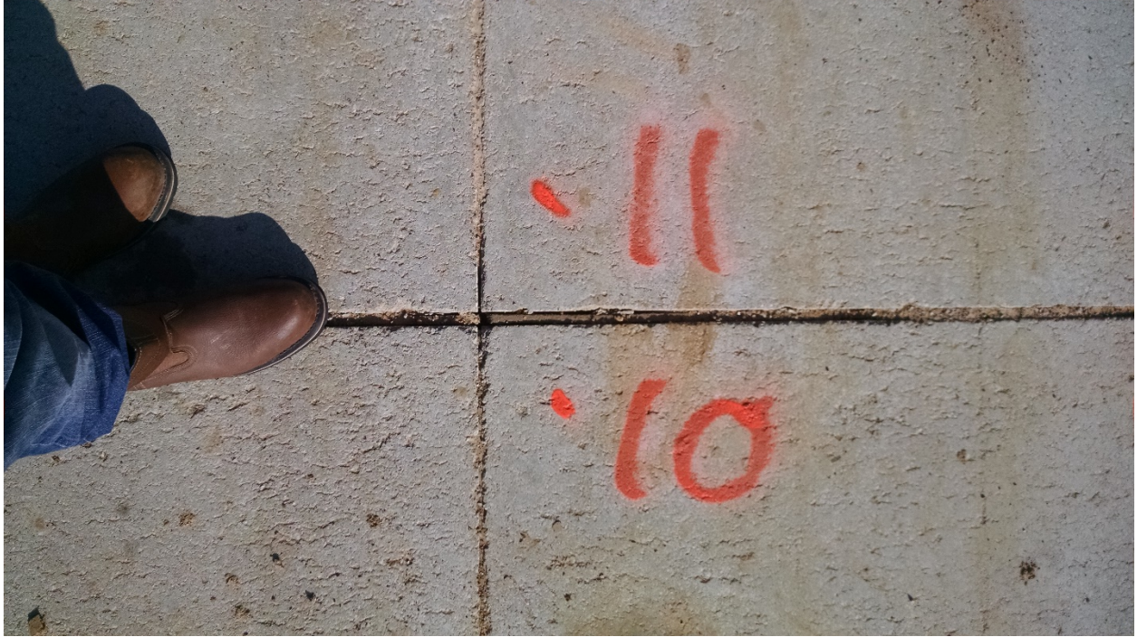
Figure 162. Bella Vista New Joint Filling with Dirt.
