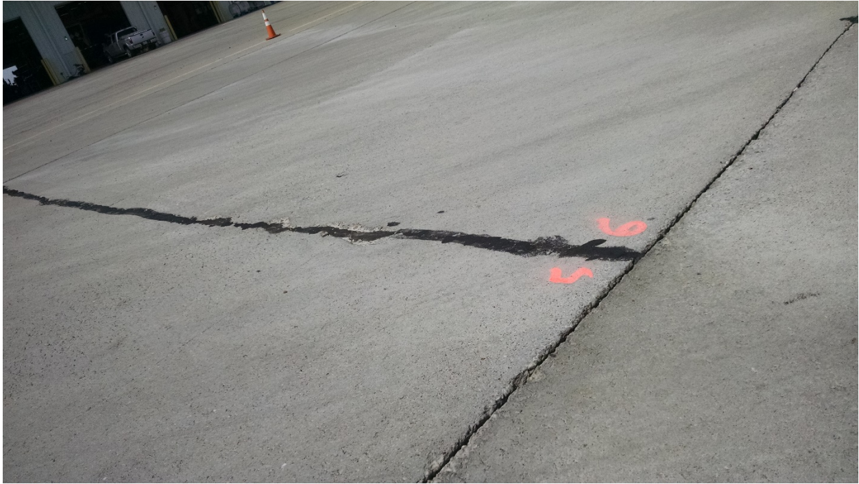
Figure 146. Pioneer Cracked Slab (Repair/Sealed with Asphalt).
