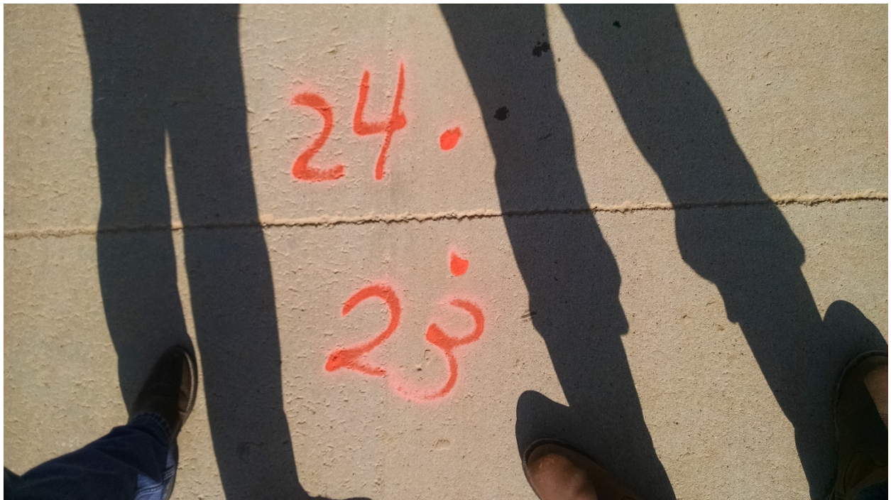
Figure 163. Bella Vista—Older Joint Already Compressed with Dirt Present.
