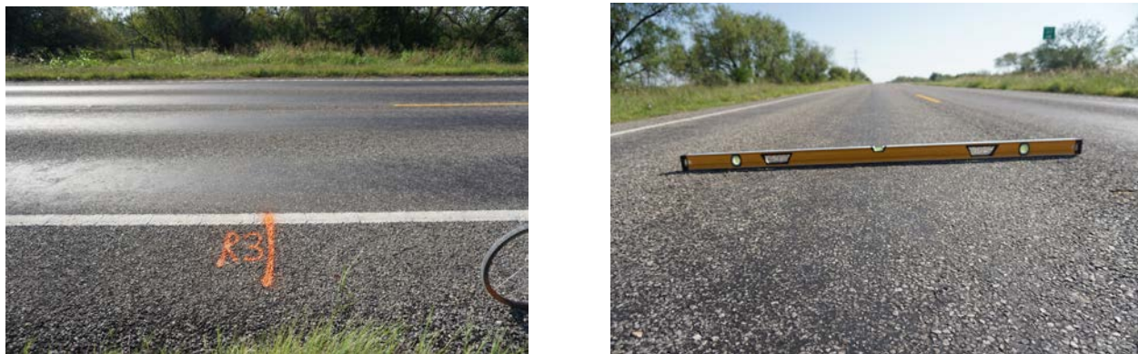
Figure 38. Pictures of Pavement Surface and Rutting: (a) No Cracking and (b) Rutting.
