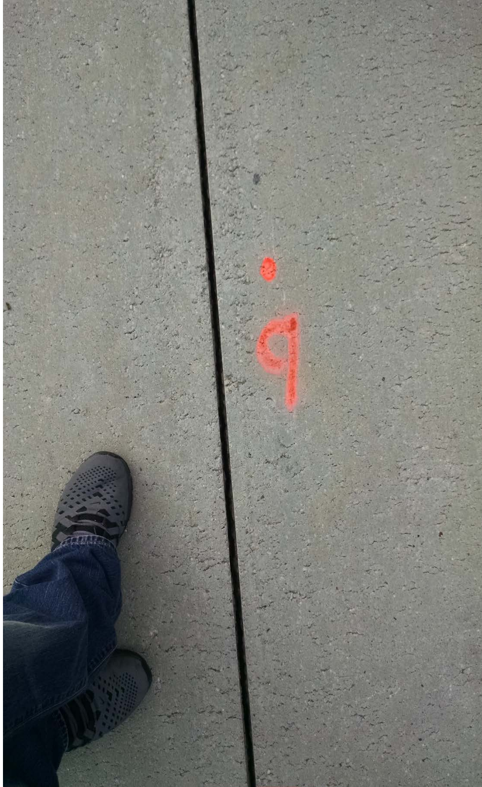
Figure 159. Bella Vista Longitudinal Joint (Separation Present) (December 2015).
