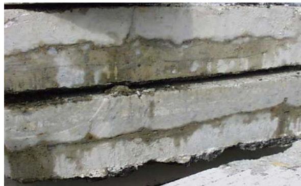
Figure 132. Formation of Deep Delamination.
