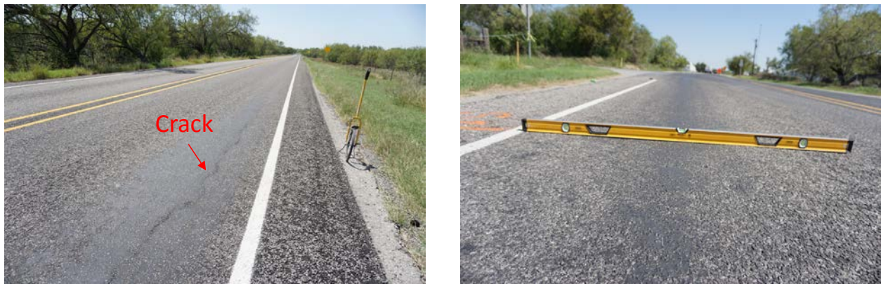
Figure 53. Pictures of Pavement Surface and Rutting: (a) Cracking and (b) Rutting.
