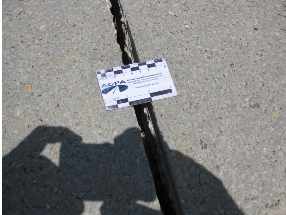
Figure 154. Bella Vista Longitudinal Joint Separation (July 2015).
