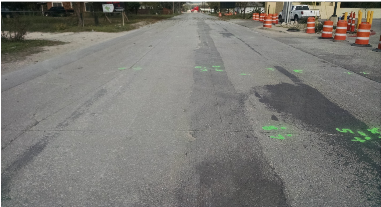
Figure 166. Solms Rd. Longitudinal Joint Spalling and Repair (along with Repair Material Failure).
