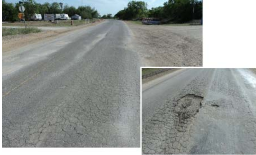
Figure 51. Condition of FM 99 prior to Rehabilitation.
