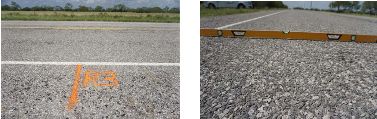
Figure 45. Pictures of Pavement Surface and Rutting: (a) No Cracking and (b) Rutting.
