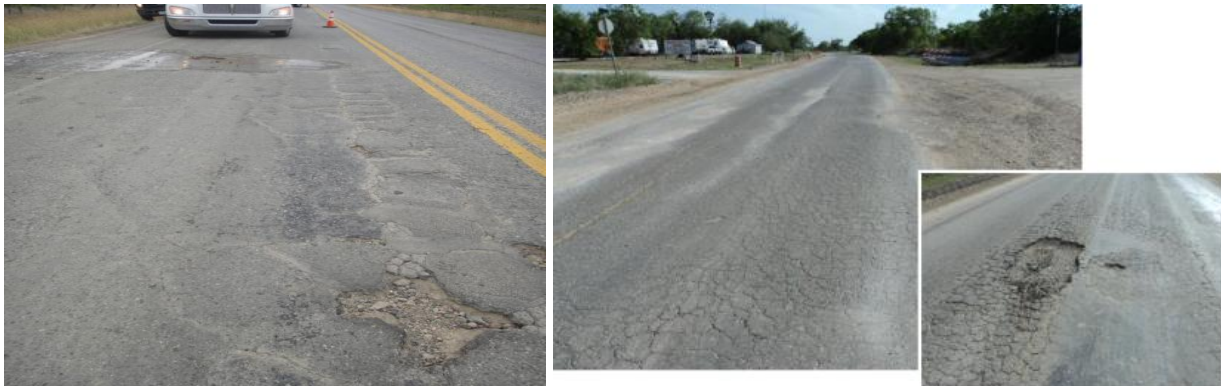
Figure 1. Pavement Damage Caused by Overloaded Trucks in Energy Development Areas.
