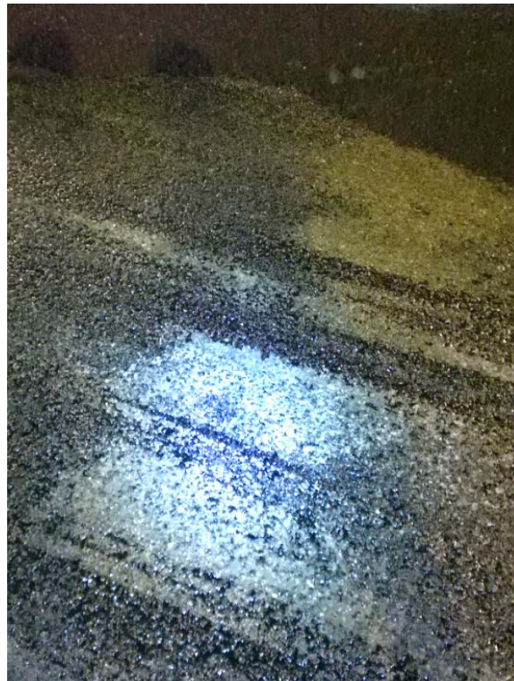
Figure 6-9. Tack Condition after Trucks Passing, RC-250 in SH 336.
