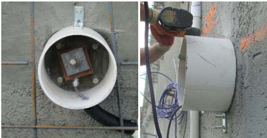
Figure 239. 12-In.-Diameter PVC Tube around the Load Cell Setup.
