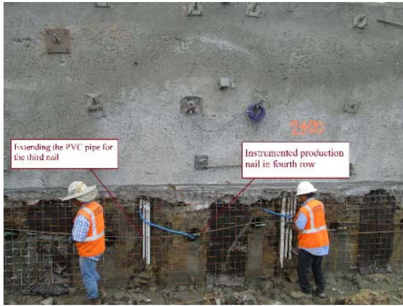
Figure 208. Extending the PVC Pipes to Conduct the Wires to the Data Acquisition System at the Fourth Stage of Construction.
