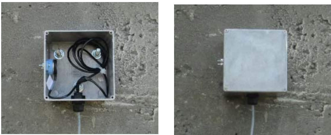
Figure 197. Aluminum Box Used to Protect Tiltmeter.
