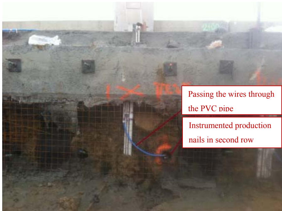
Figure 207. Extending the PVC Pipes to Conduct the Wires to the Data Acquisition System at the Second Stage of Construction.
