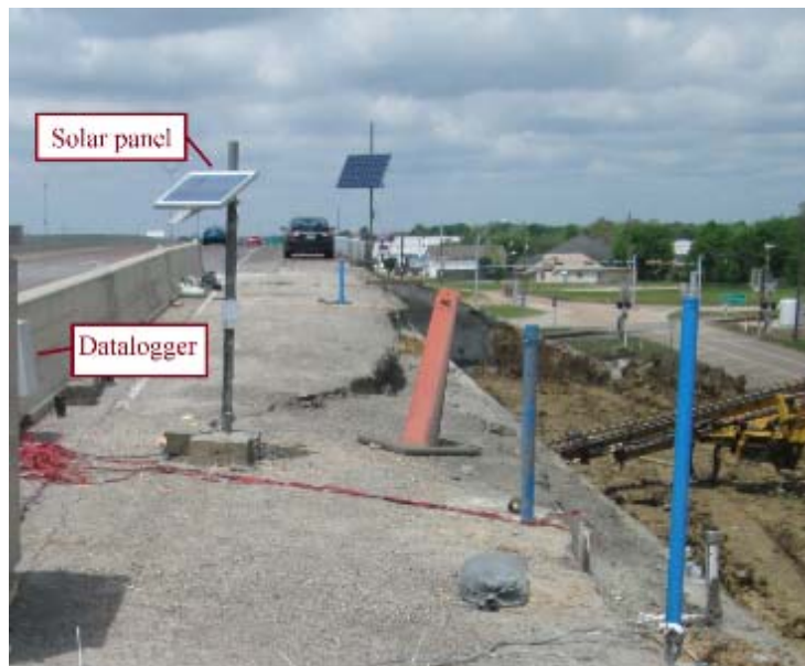
Figure 220. Solar Panel Installed next to the Data Logger at the Temporary Location at Station 2+00.
