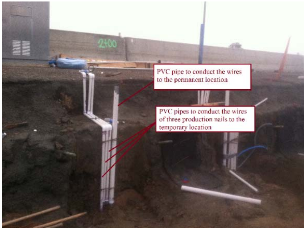
Figure 206. Location of the PVC Pipes to Conduct the Wires from the Strain Gauges to the Data Acquisition System, First Stage of Construction.
