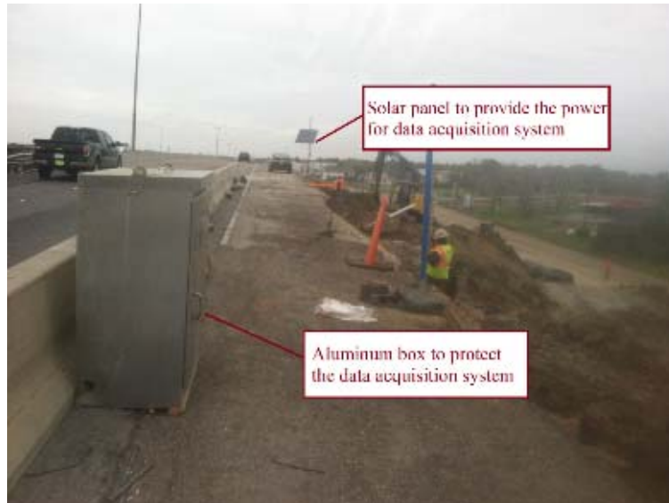
Figure 202. Temporary Location of the Data Acquisition System and Solar Panel.
