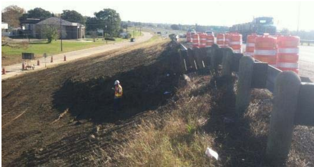
Figure 149. View of the Embankment before the Project Was Started (the Soil Was Unstable and Failed at the Section Next to the Bridge).
