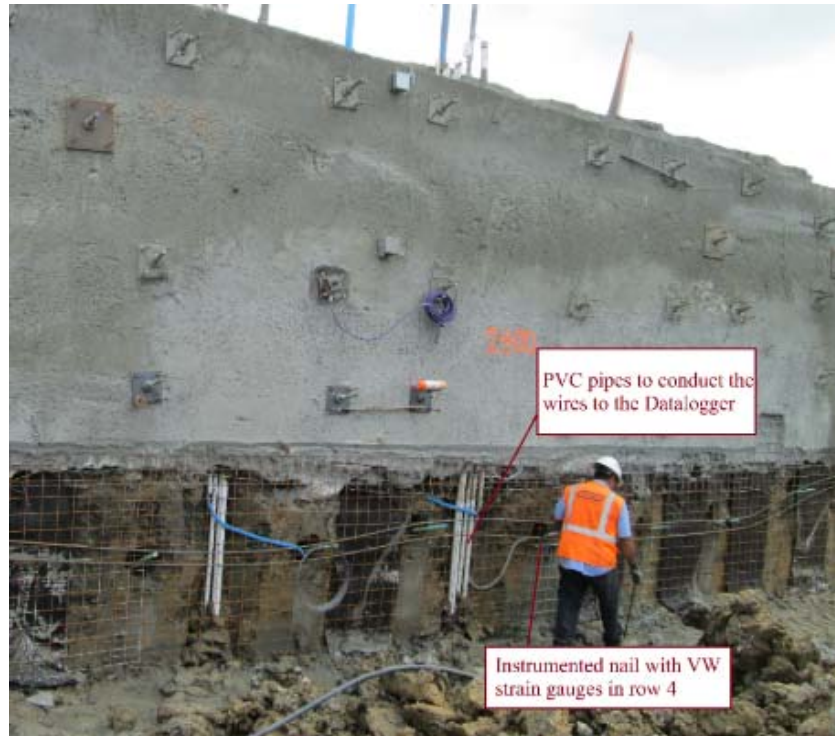
Figure 224. PVC Pipes to Conduct the Wires to the Data Logger at Fourth Stage of Construction at Station 2+00.
