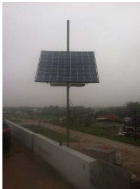
Figure 203. Solar Panel for Providing Power for Data Acquisition System.
