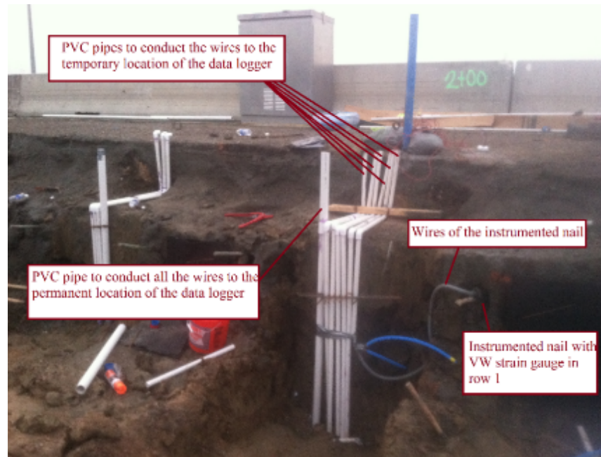
Figure 223. PVC Pipes to Conduct the Wires to the Data Logger at First Stage of Construction at Station 2+00.
