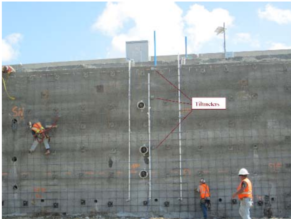
Figure 198. Three Tiltmeters Installed at Different Depths of the Wall.
