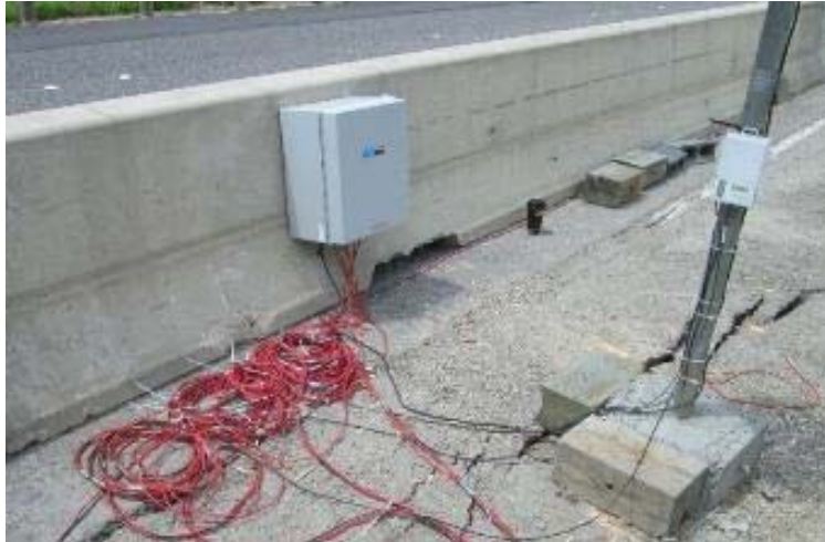
Figure 219. Data Logger Box at the Temporary Location Top of the Wall at Station 2+00.
