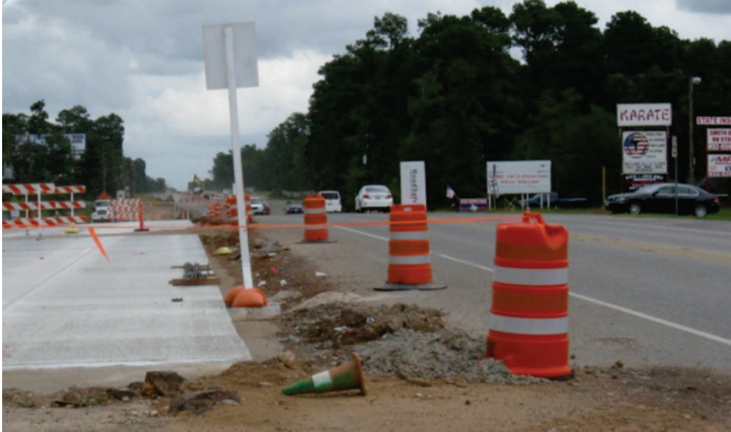
Figure 2. Driver's View from a Passenger Car in a Driveway in a Texas Work Zone (3).
