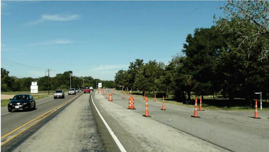
Figure 4. Multiple Driveways with 42-Inch Tall Cones in a Rural Area.
