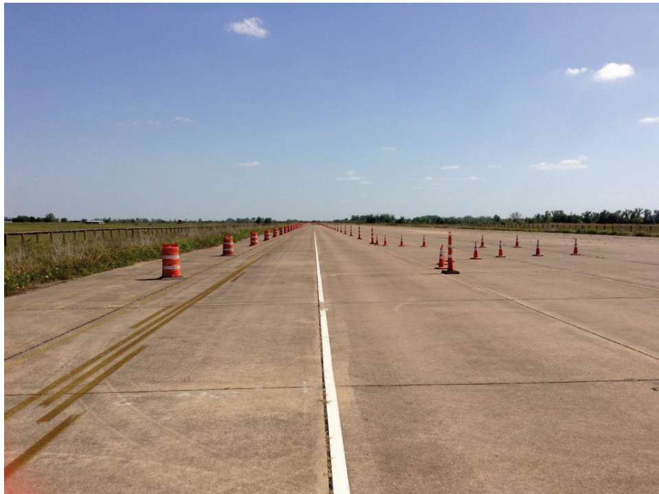
Figure A-24. Treatment 2: 42-Inch Cones on Main Lane with 28-Inch Cones on Driveway.
