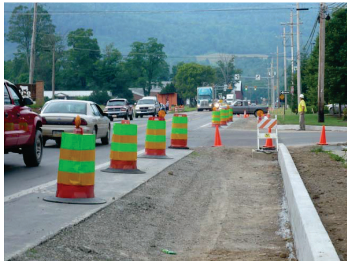
Figure 9. Green and Yellow Striped Channelizing Drums Used in PennDOT Research.
