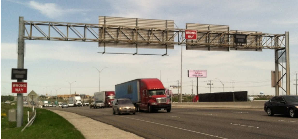
Figure 40. Example of Installed Mainlane System.
