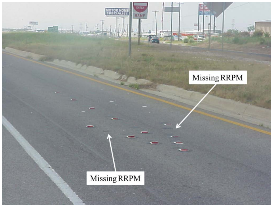
Figure 30. Example of Missing RRPMs in a Wrong Way Arrow.
